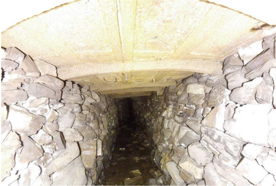
Rusted steel doors 30 ft of Entry 6
