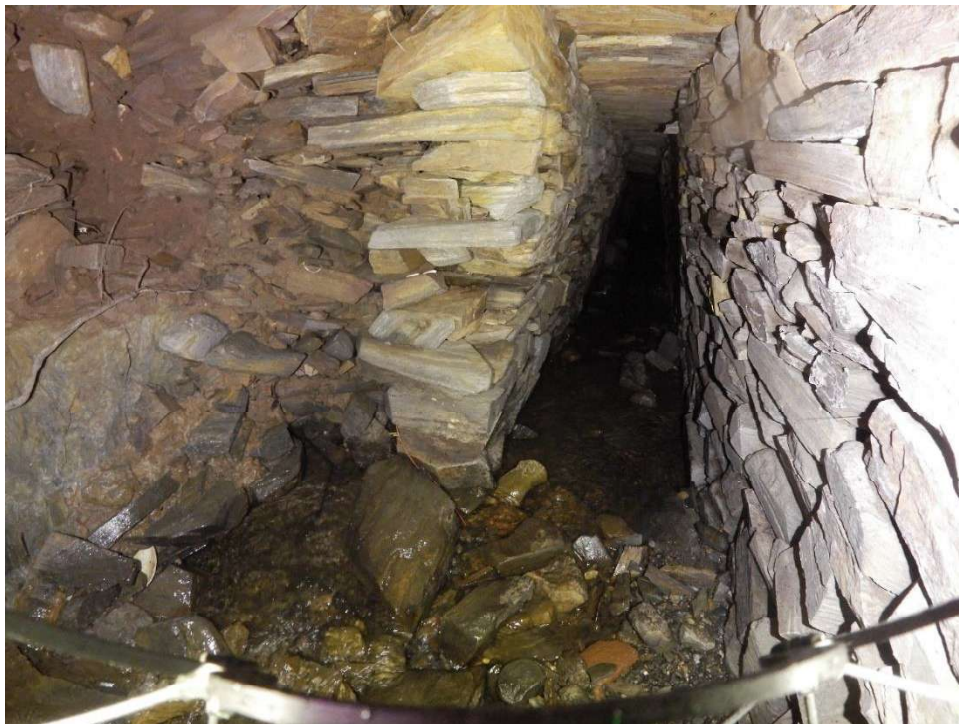
Major stone tunnel collapse 65 ft from Entry 10
