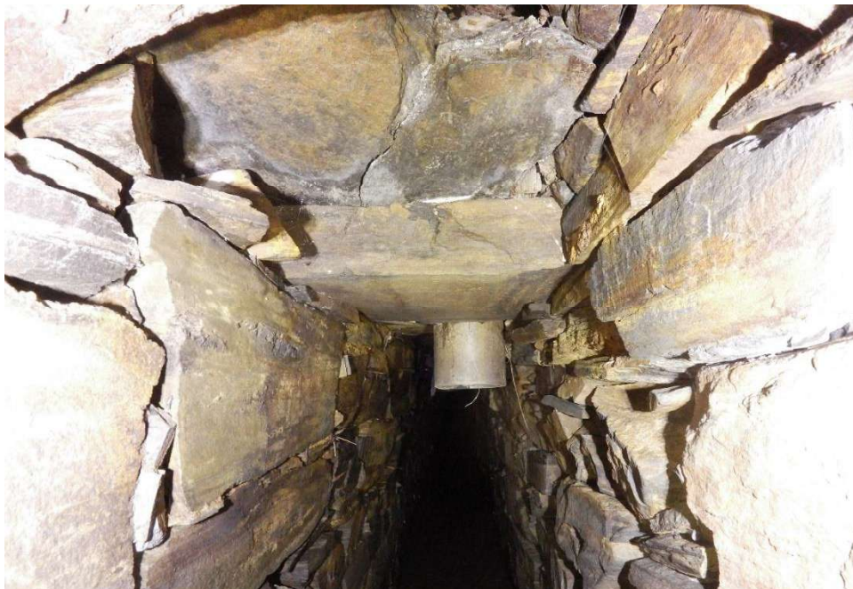
Crack on ceiling 75 ft from Entry 7
