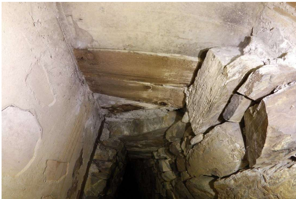
Moist timber with water stains on ceiling 36 ft from Entry 10
