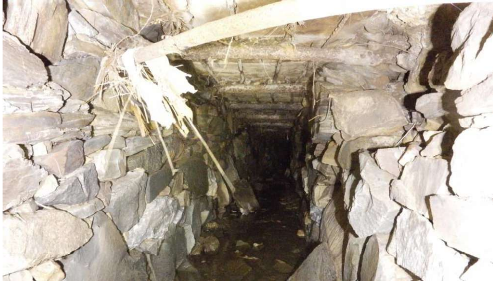
Minor rock collapse about 40 ft from Entry 1
