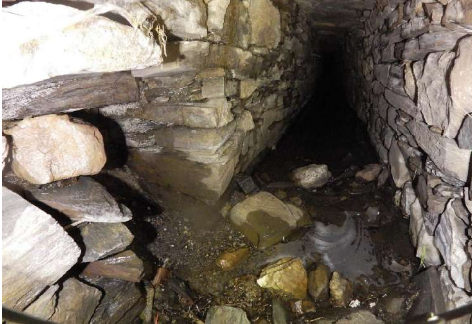
Minor rock collapse 65 ft from Entry 3
