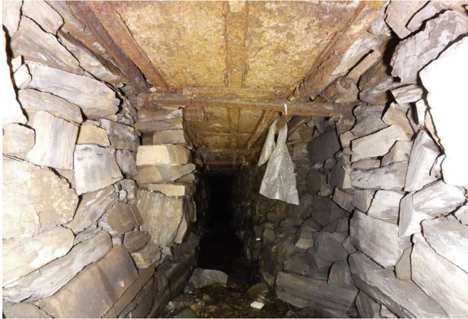
Rusted steel doors 1 ft from Entry 7
