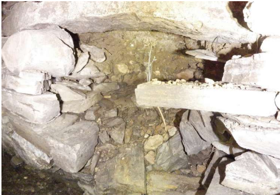
Minor rock collapse 20 ft from Entry 2
