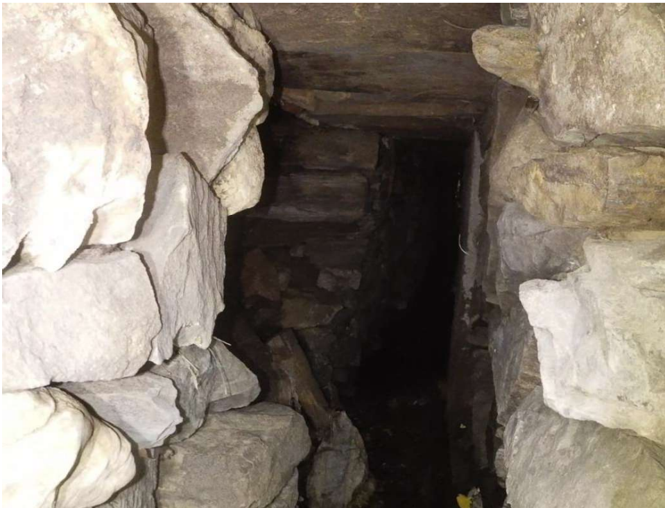
Minor rock collapse 85 ft from Entry 5
