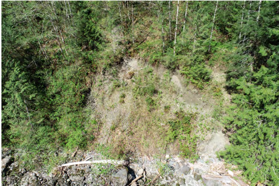
PHOTO 3: Steep slope below pipeline alignment near STA 42+50. Pipeline is about 11 feet upslope from head scarp. View from UAV to the west.
