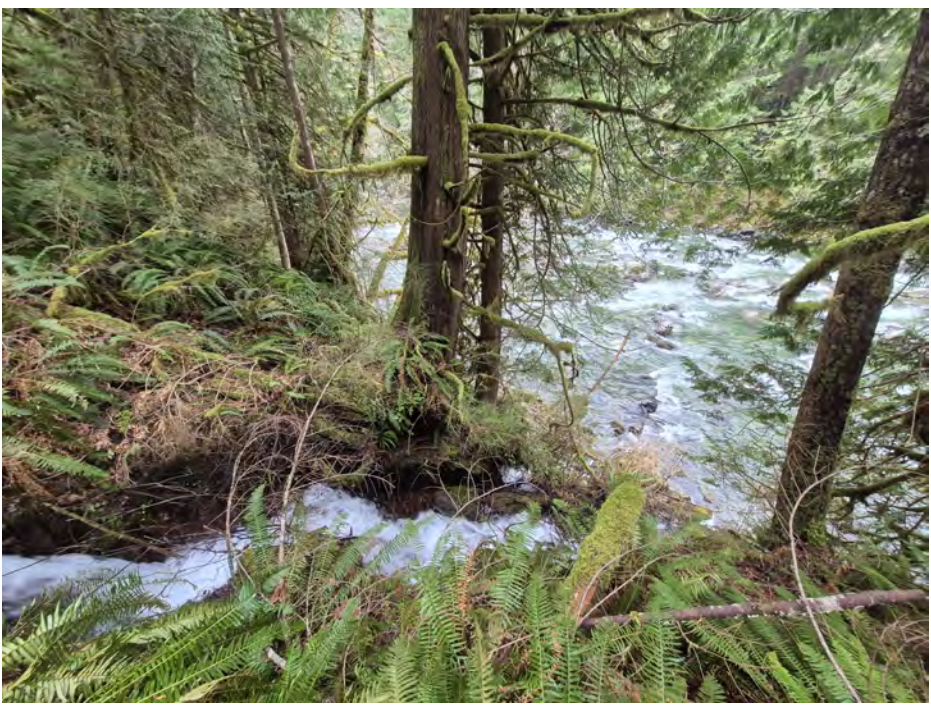
PHOTO 6: Gully incising into slope below trail at culvert outlet near STA 52+00. View downslope and to the southeast.
