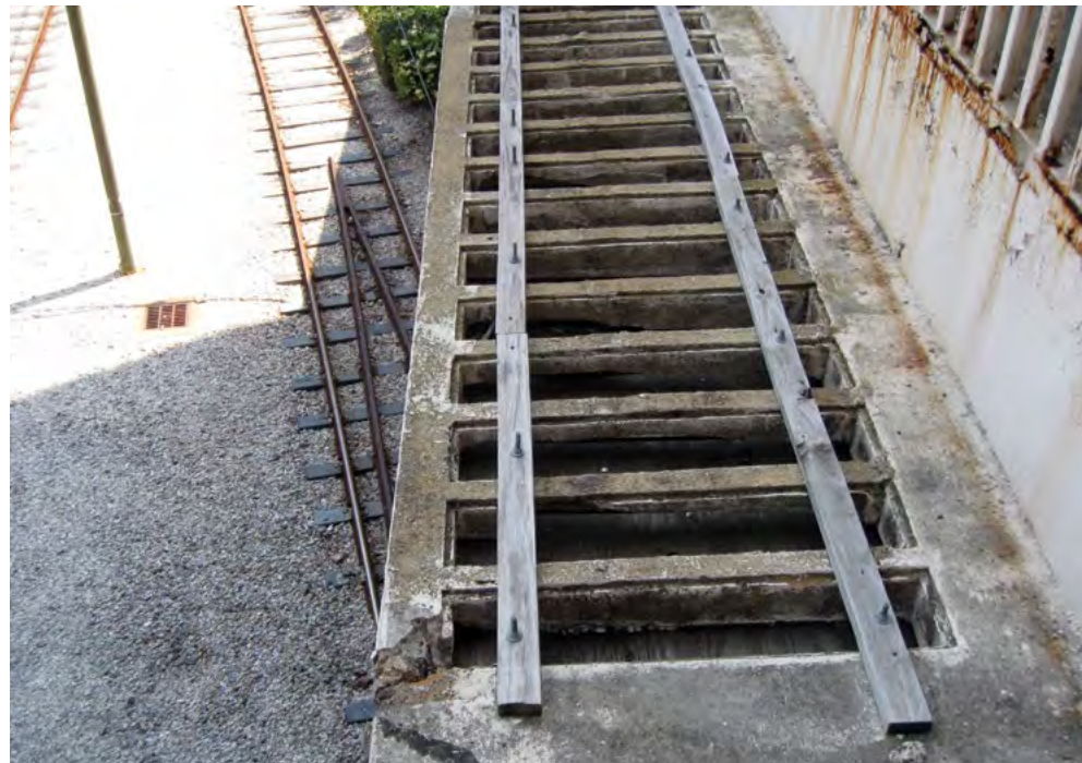
[6] Some areas of the concrete brise soleil screen on this building constructed in 1967 are badly deteriorated. If the screen cannot be repaired, it may be replaced in kind or with a composite substitute material with the same appearance as the concrete.
