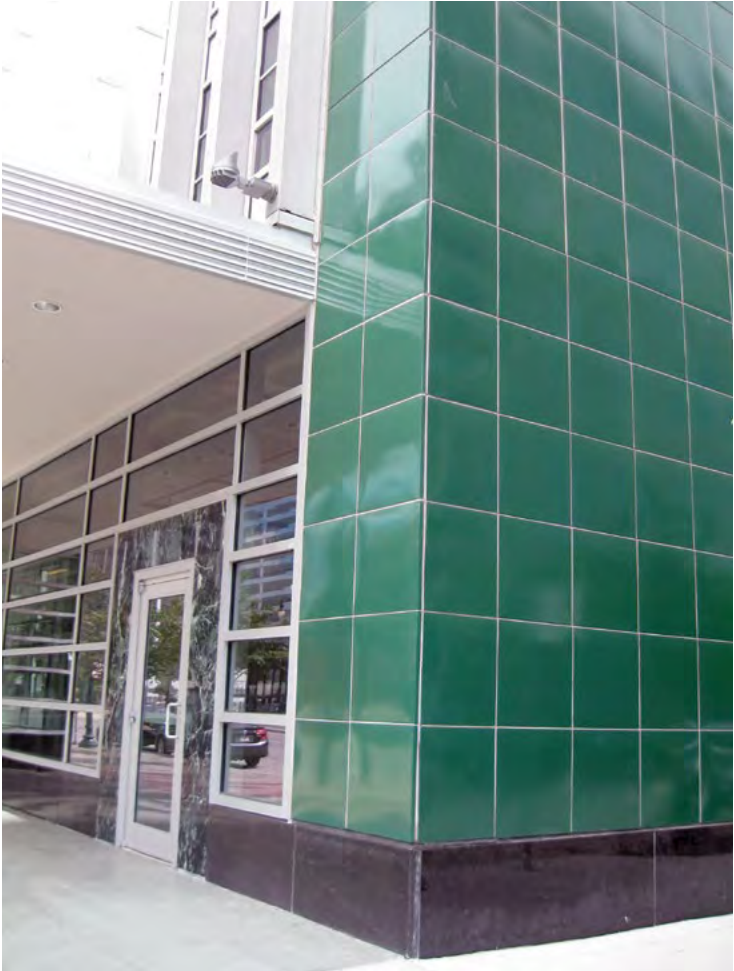
[15] New enameled-metal panels were replicated to replace the original panels, which were too deteriorated to repair, when the storefront of this early 1950s building was recreated.
