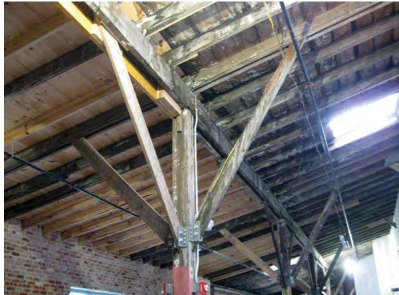
[17] New wood elements have been used selectively to replace rotted wood on the underside of the roof in this historic warehouse.
