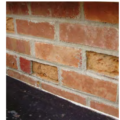
[2] Not Recommended: The use of inappropriate Portland cement mortar to repoint these soft 19th-century bricks has caused some of them to spall. Photo: Courtesy Nebraska State Historic Preservation Office.
