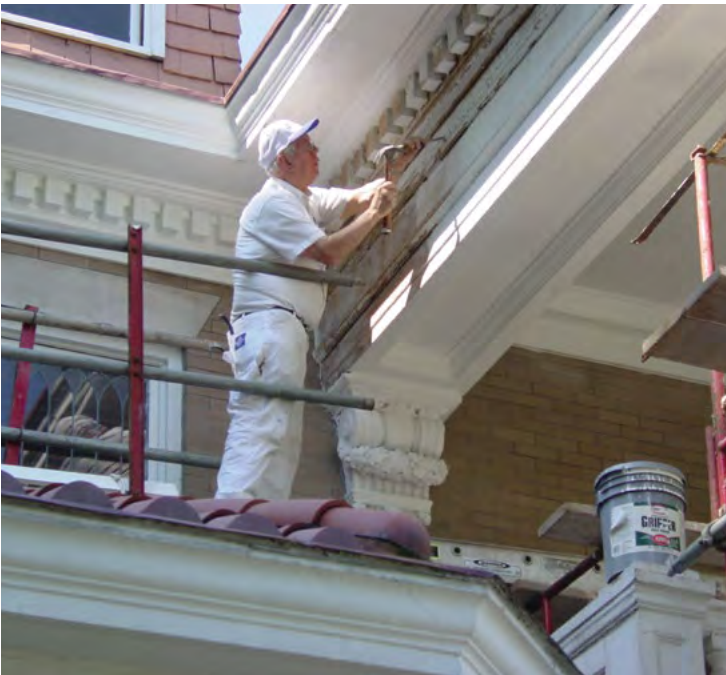
[12] Repair and limited replacement in kind to match deteriorated wood porch features is always a recommended preservation treatment.
