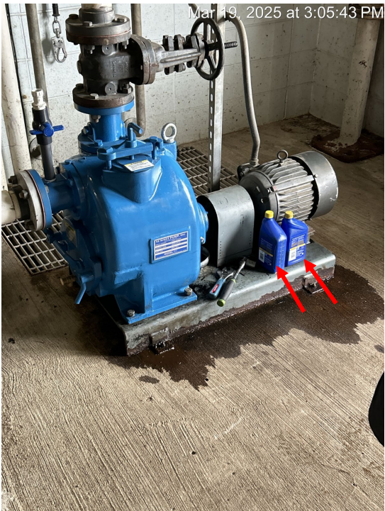
Photograph 12. Breezeway pumping building, northern pump leaking oil, containers without secondary containment indicated by red arrows.
