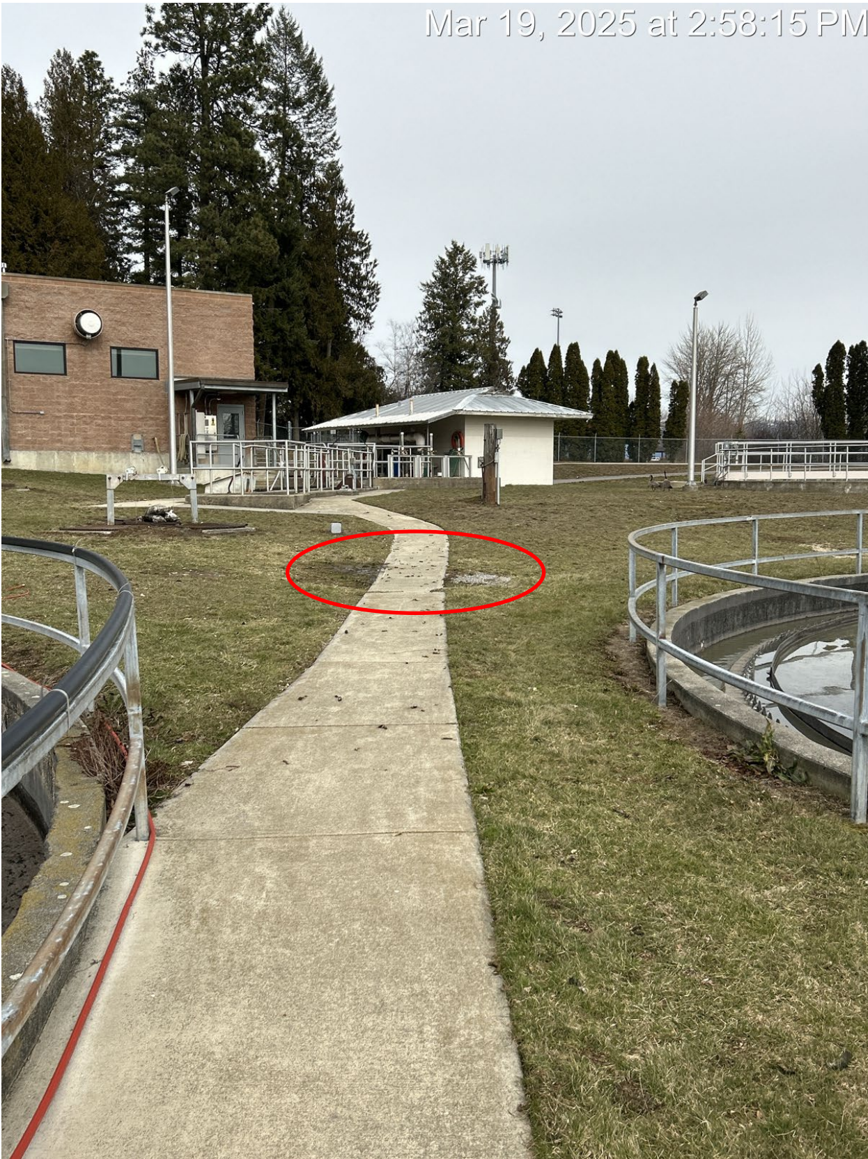
Photograph 13. Pipe leak between headworks and primary clarifiers indicated by a red circle, facing northeast.
