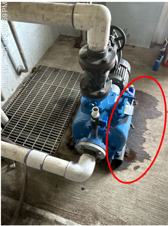
Photograph 11. Breezeway pumping building, oil bordering northern pump indicated by a red circle.
