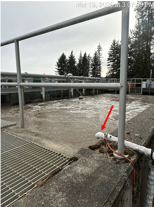
Photograph 5. Aeration basin overview with groundwater pipe discharging to the basin indicated with red arrow, facing southwest.
