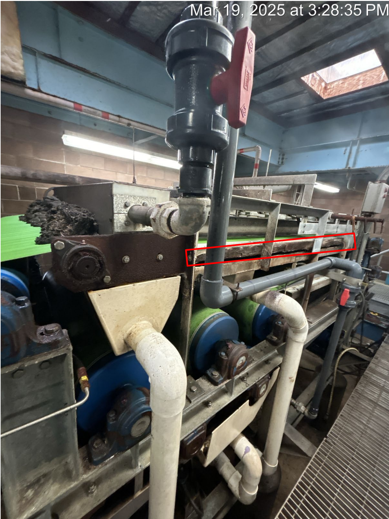
Photograph 9. Belt press overview, deteriorated portion outlined by a red box.
