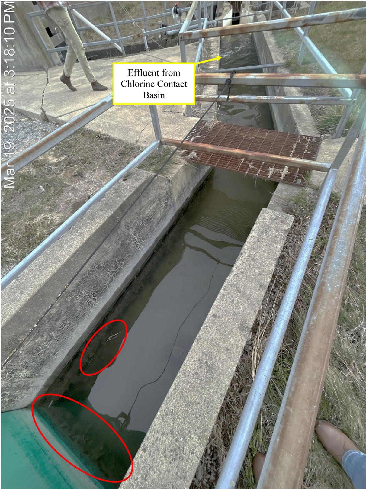
Photograph 10. Upstream of chlorine contact chamber effluent to receiving waters, algae and debris indicated by red circles, facing southeast.
