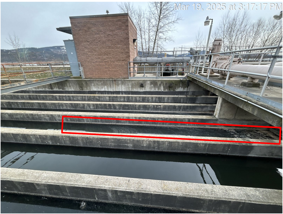
Photograph 7. Chlorination contact chambers, red box indicating floating solids facing southeast.
