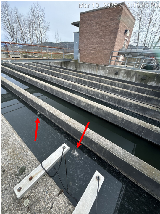
Photograph 6. Chlorination contact chambers, red arrows indicating floating solids, facing east.
