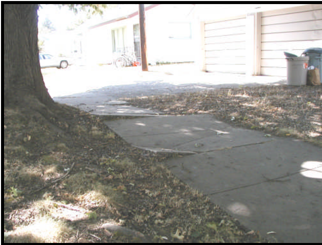
Figure 23: A sidewalk being lifted by roots
