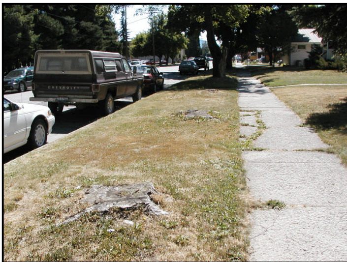
Figure 20: Stump removal results in nicer-looking plant strips that are free of tripping hazards and have more room to plant new trees.
