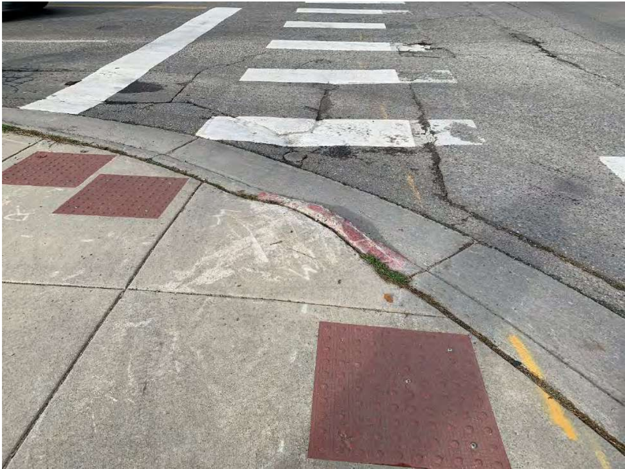
Observation 3: Non-ADA-compliant pedestrian ramps and crosswalks (Photo: Fehr & Peers).
