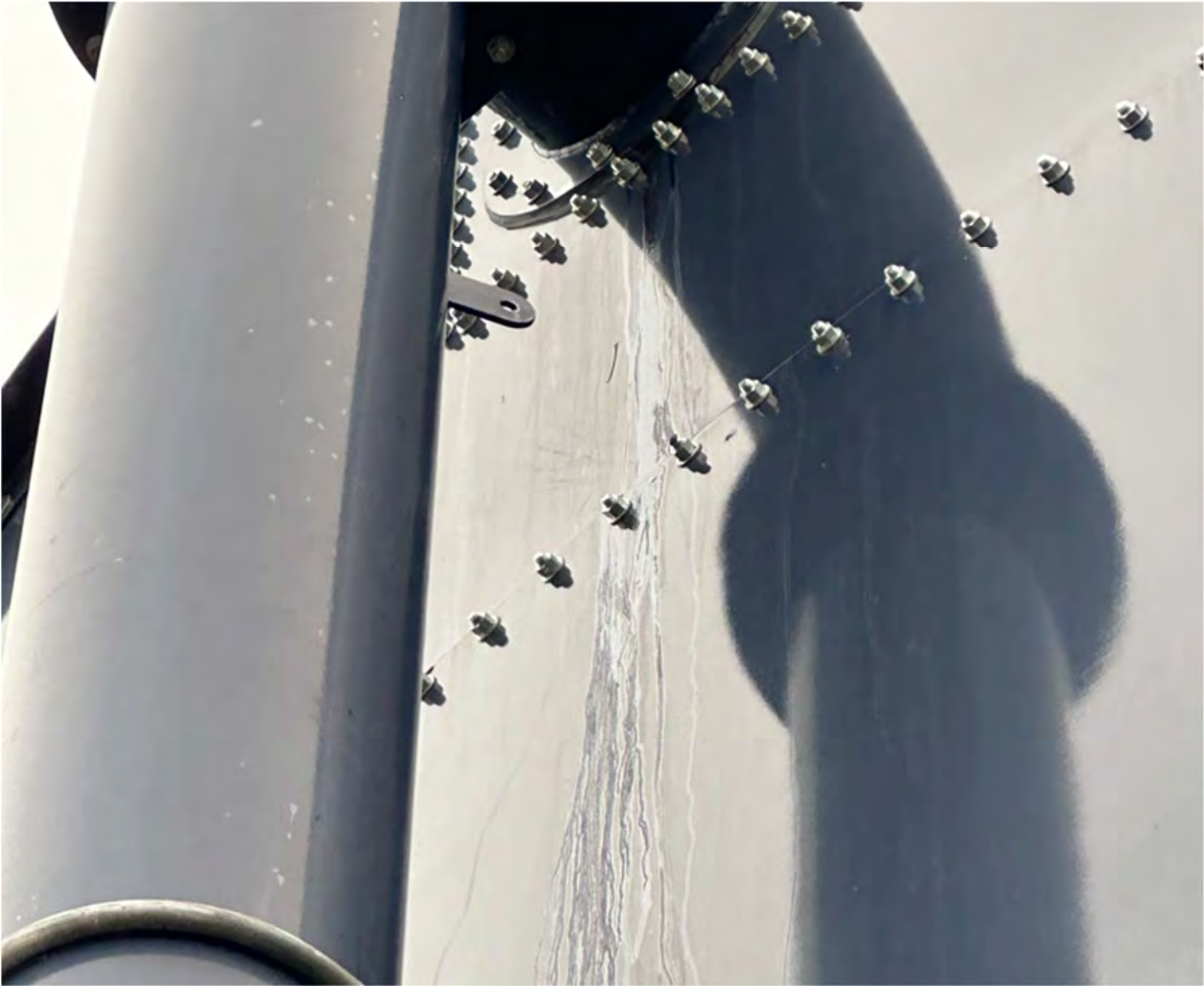
FIGURE 12 - LEAK 12, OVERFLOW PIPE
