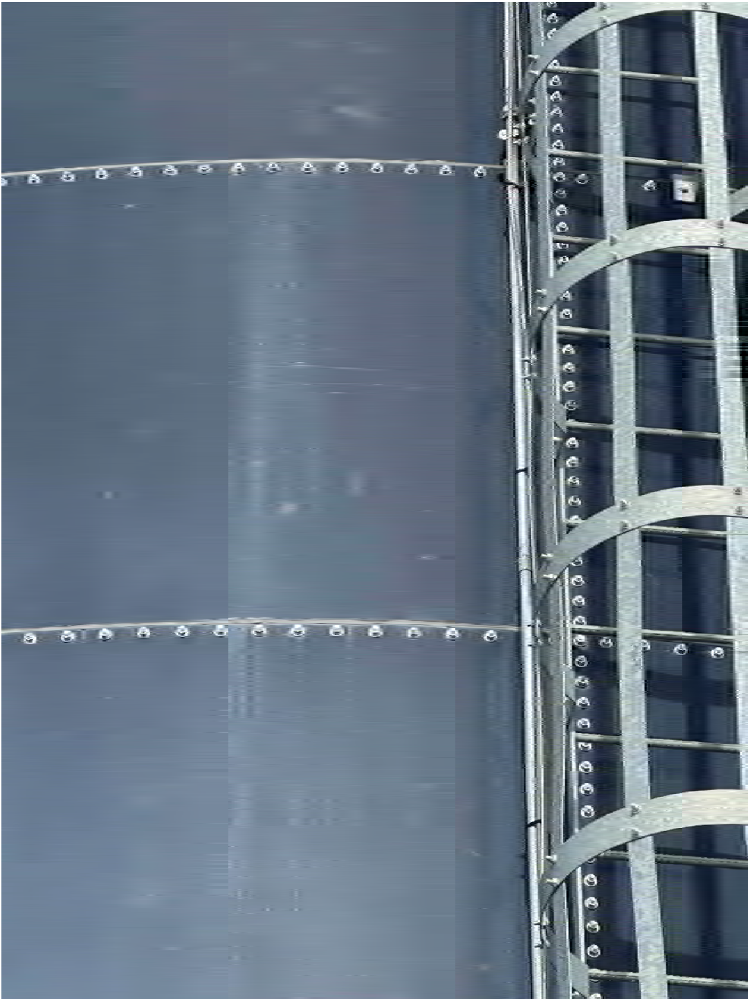
FIGURE 11 - LEAK 11, NEW LEAK FROM BOLTS
