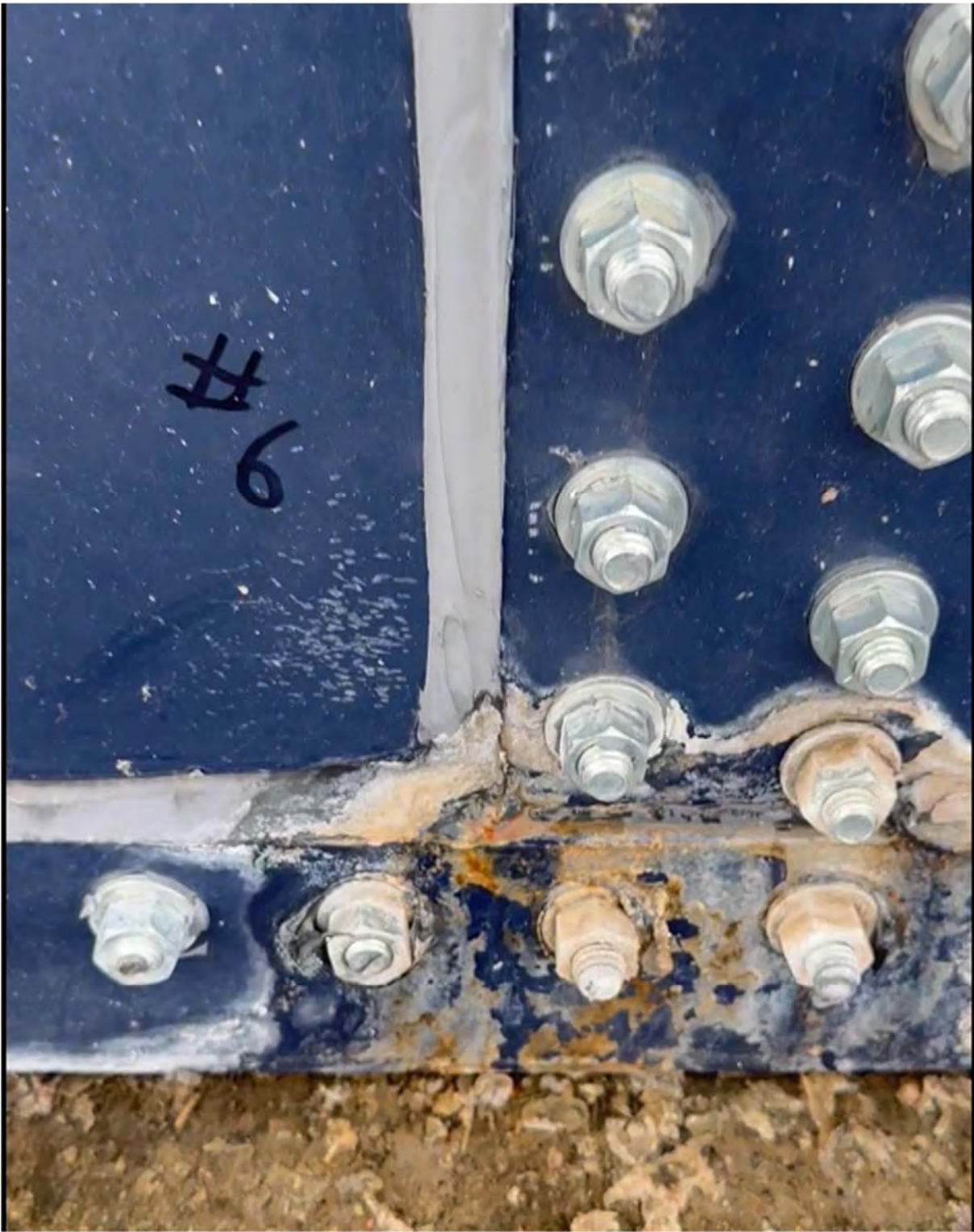
FIGURE 6 - LEAK 6, FLOWING LEAK
