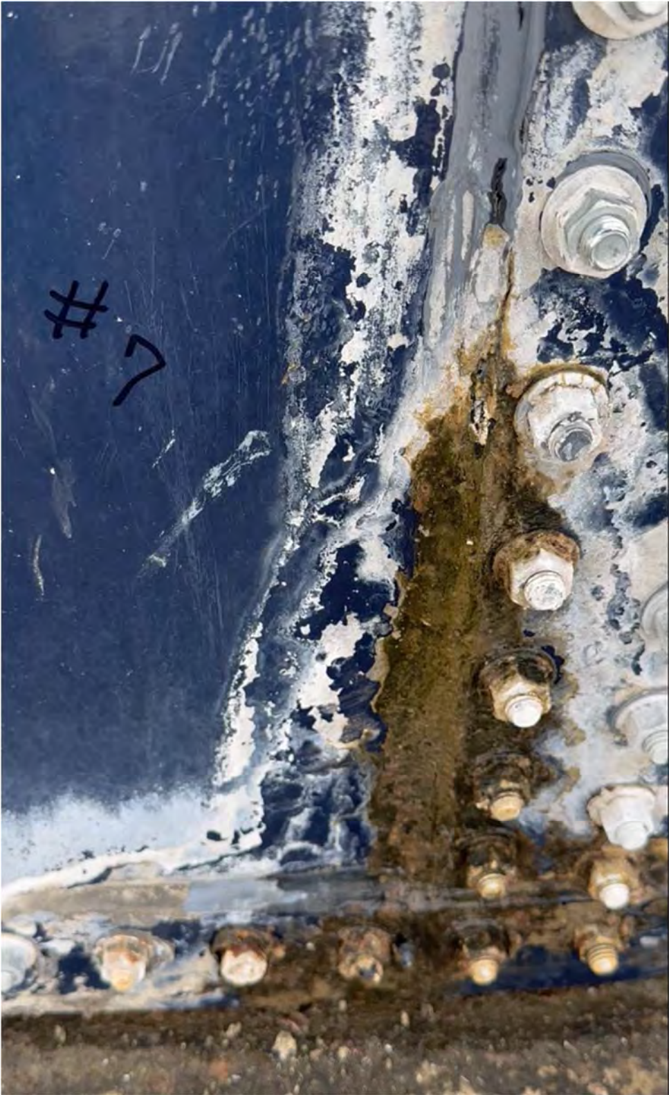
FIGURE 7 - LEAK 7, LEAK AT SEAM
