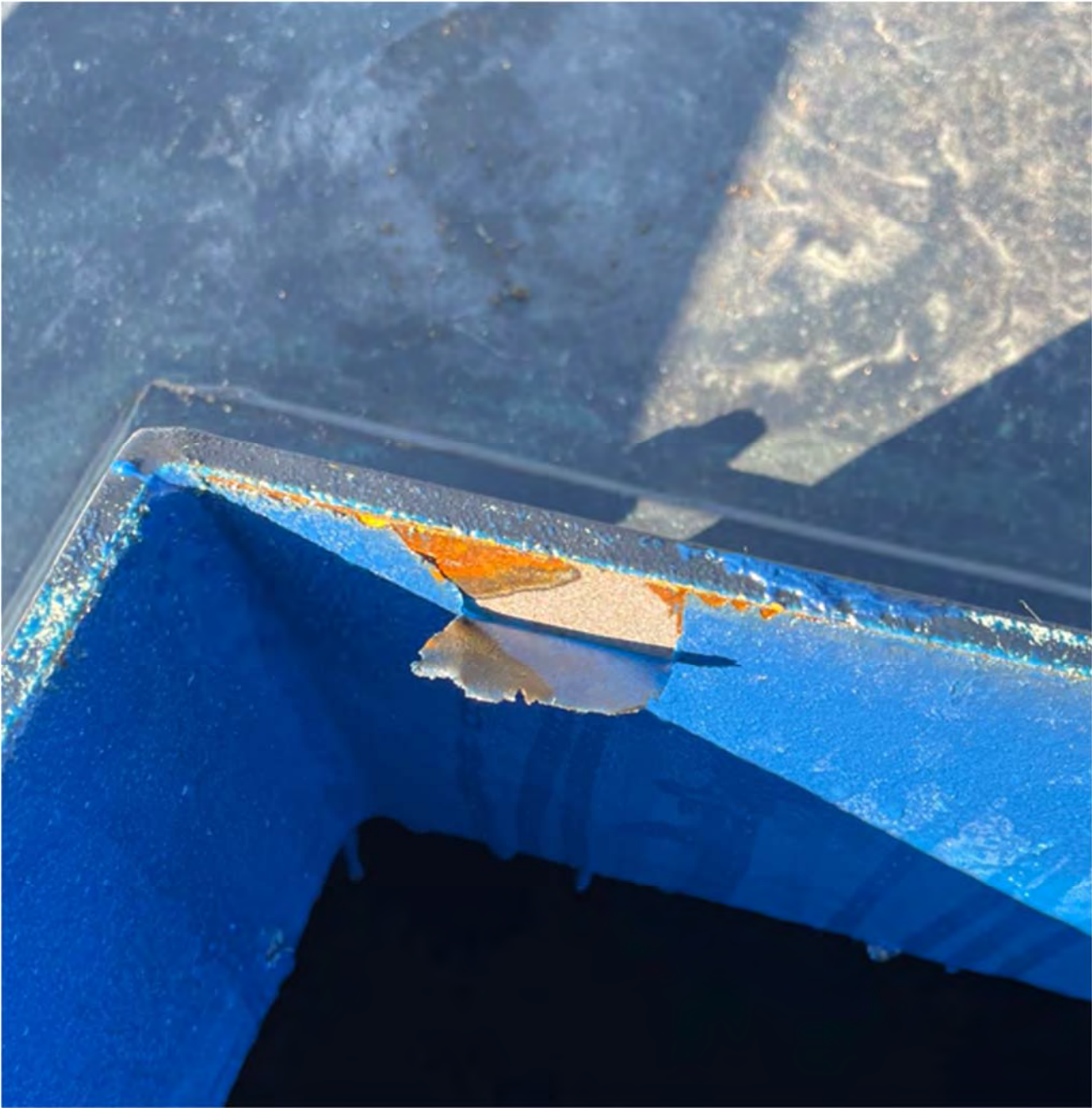
FIGURE 15 - PEELING LINER, UPPER HATCH RIM
