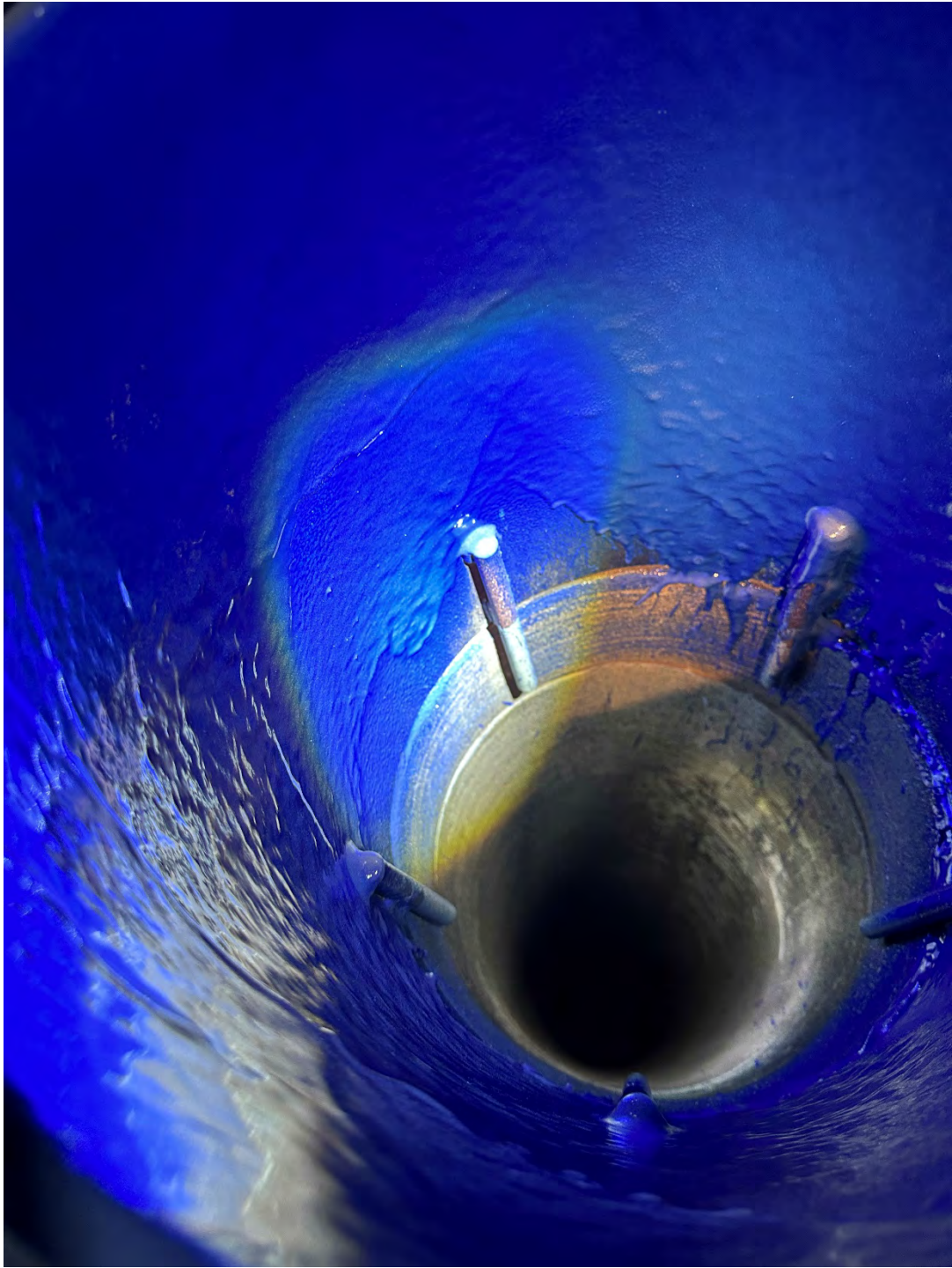
6. Areas on floor show loose caulk around bolts.
