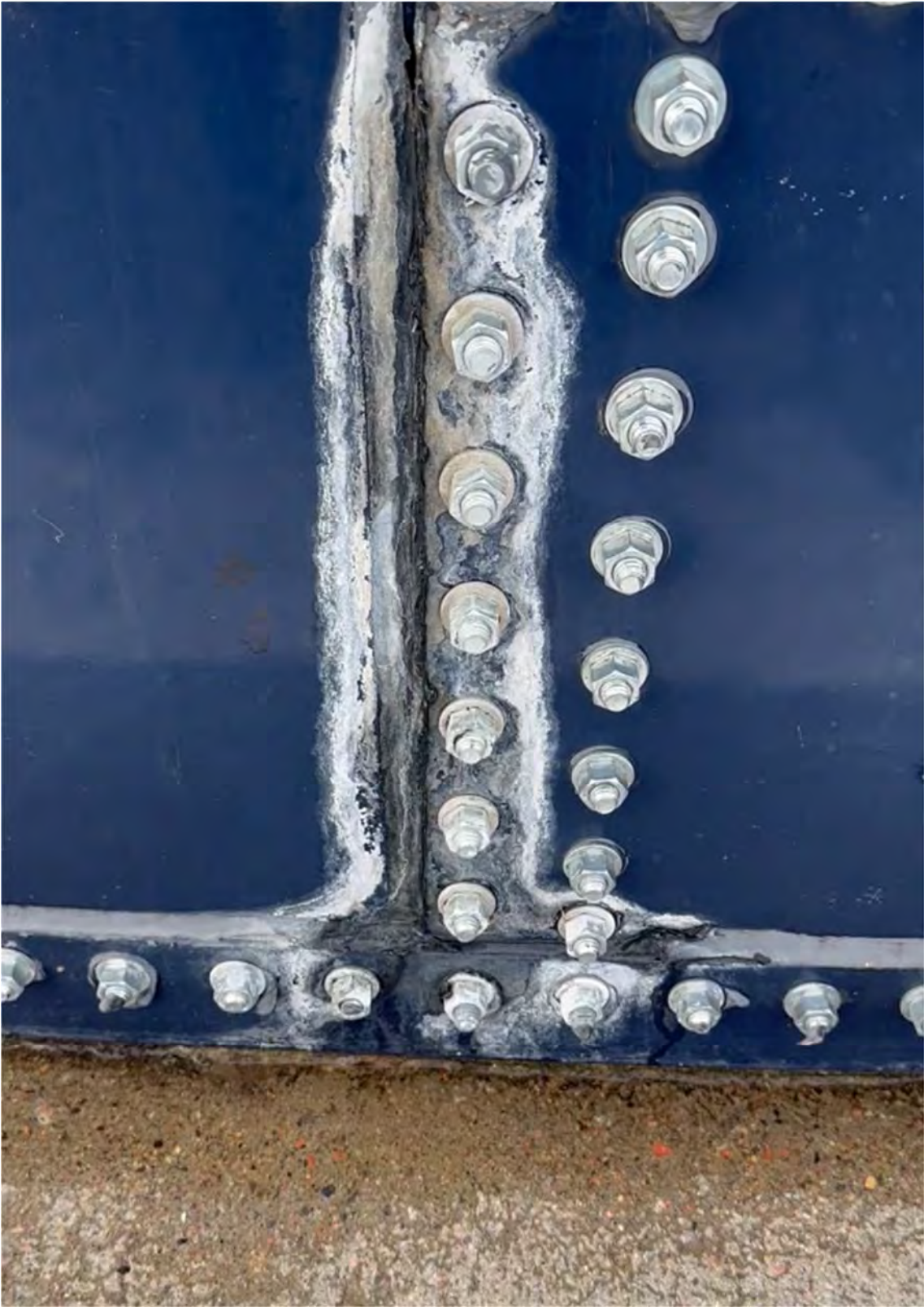
FIGURE 5 - LEAK 5, LOCATION OF PREVIOUS AND EXISTING LEAK
