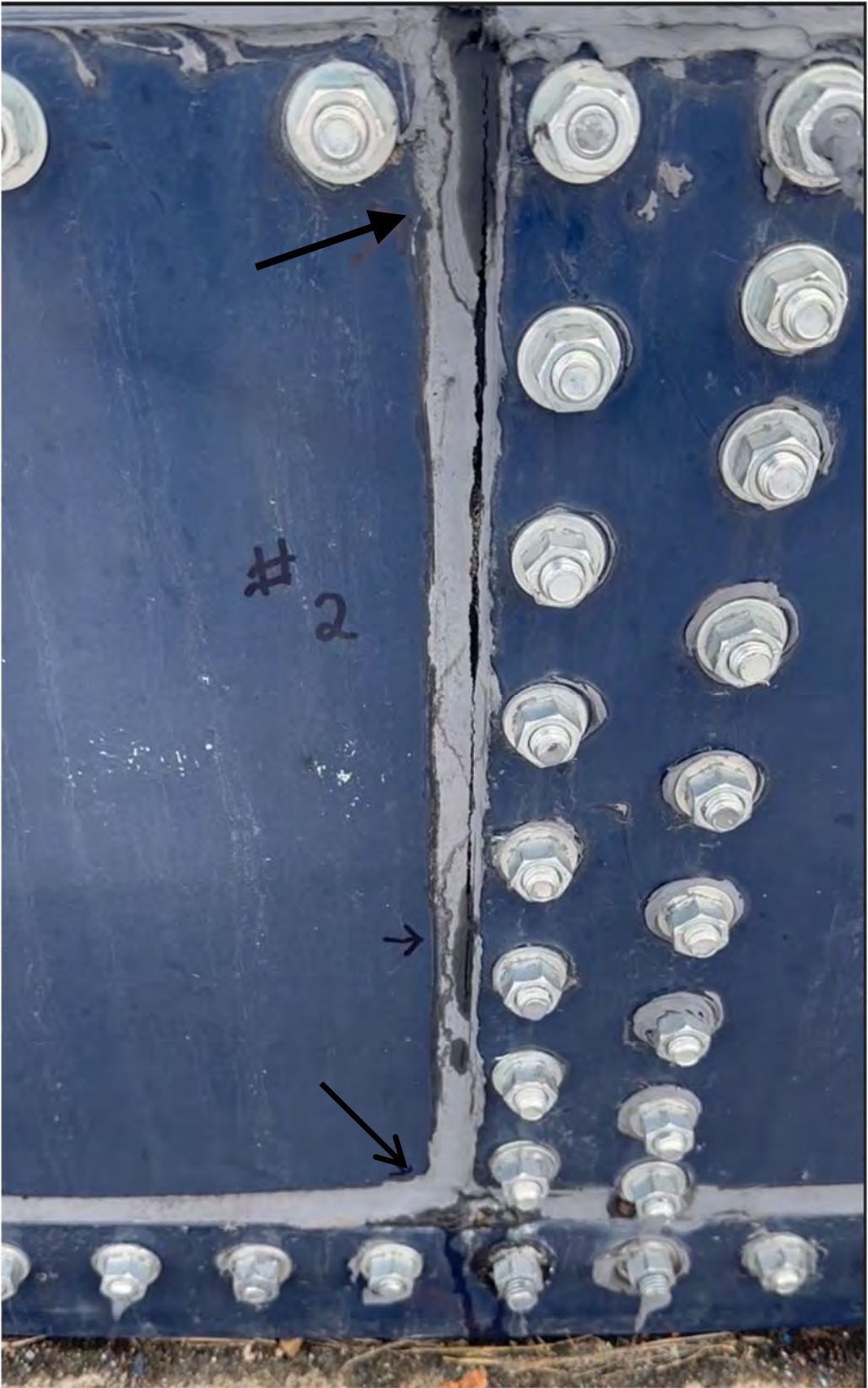
FIGURE 2 - LEAK 2, NEW LEAK APPEARED AFTER LINING
