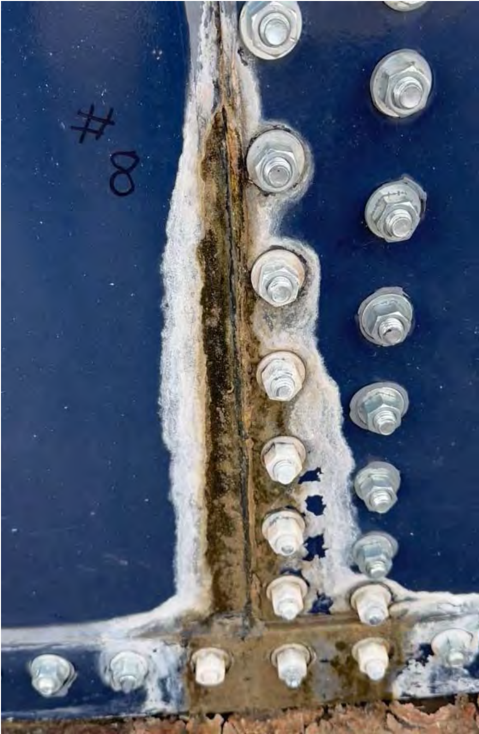
FIGURE 8 - LEAK 8, PREVIOUS AND EXISTING LEAK
