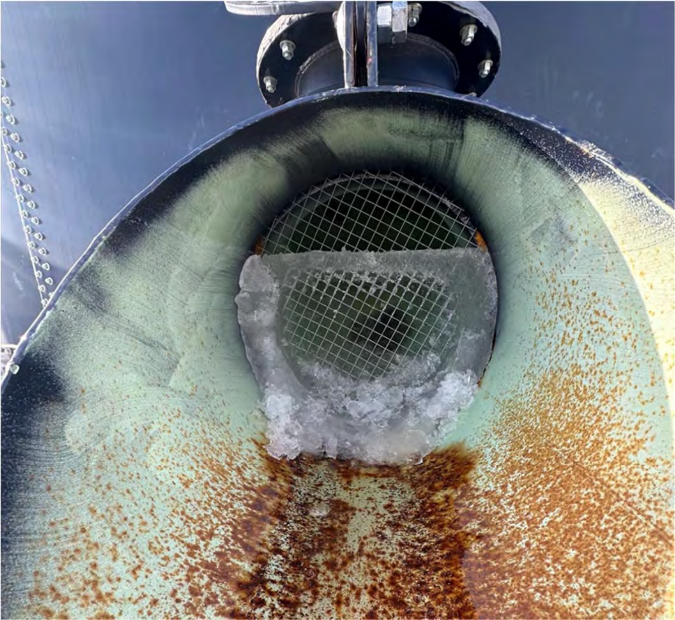
FIGURE 14 - OVERFLOW PIPE OUTLET ICE BUILDUP
