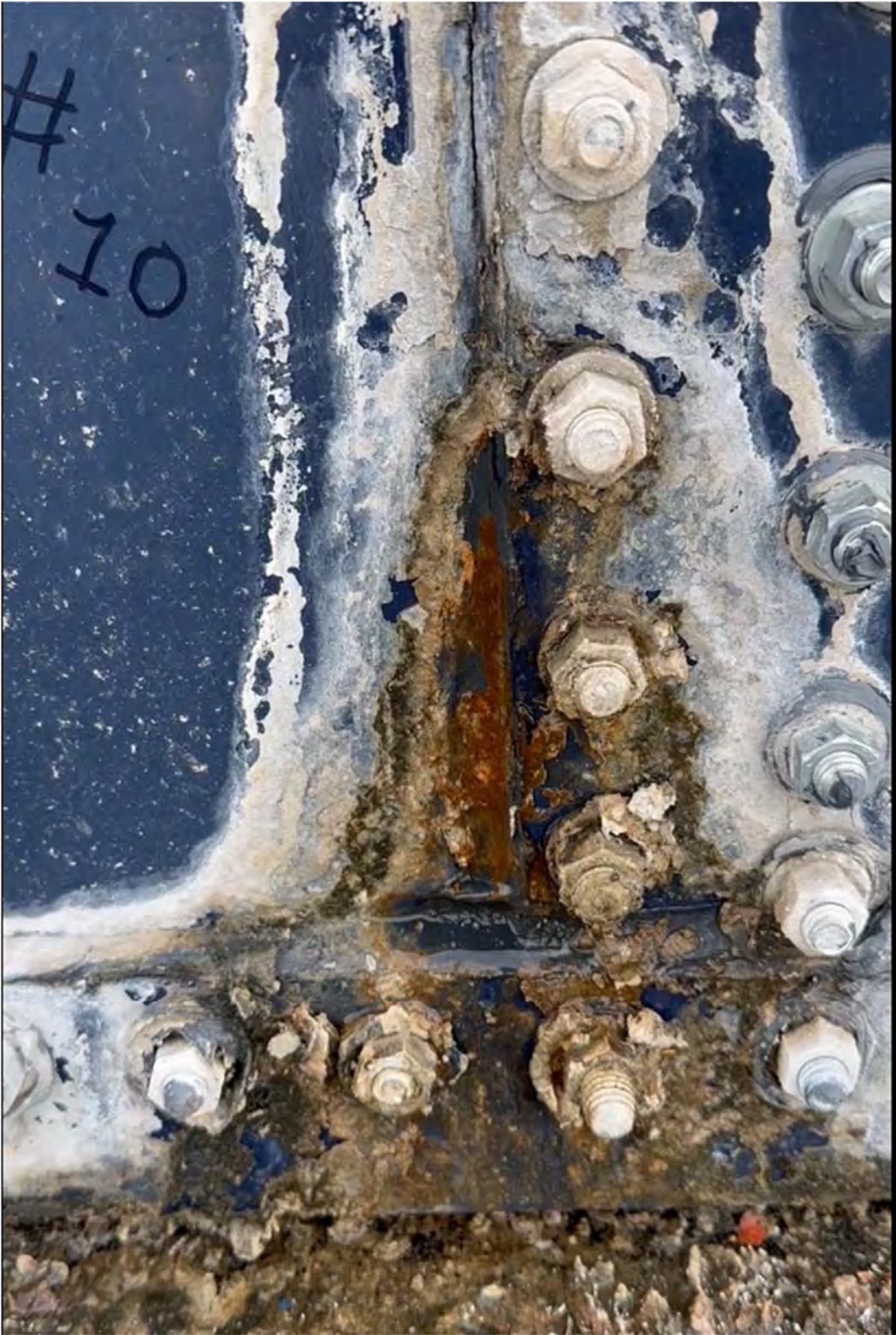
FIGURE 10 - LEAK 10, PREVIOUS AND EXISTING LEAK
