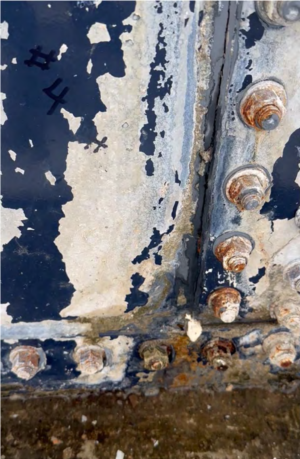
FIGURE 4 - LEAK 4, LOCATION OF PREVIOUS AND EXISTING LEAK
