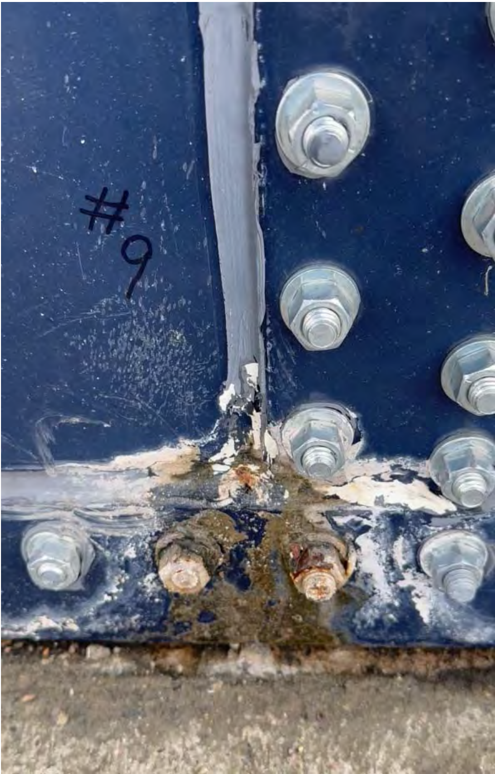
FIGURE 9 - LEAK 9M PREVIOUS AND EXISTING LEAK AT FLANGE SEAM.
