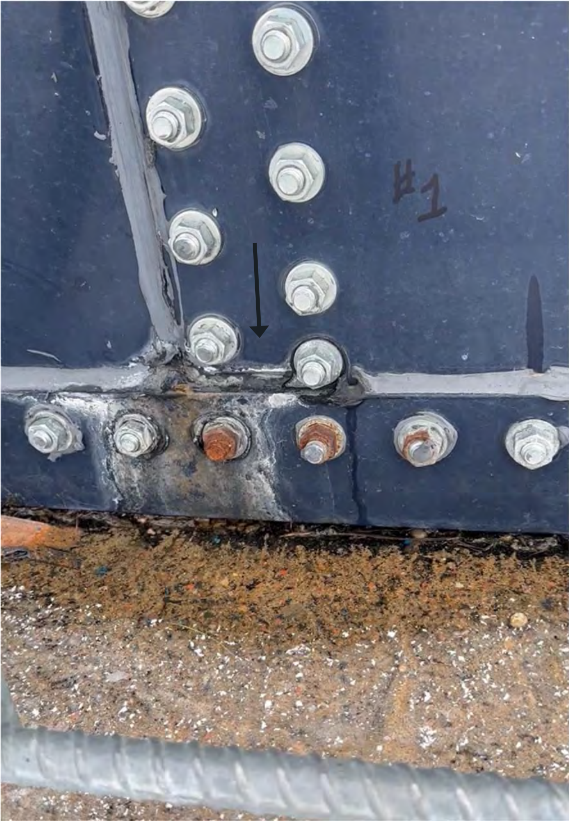
FIGURE 1 - LEAK 1, LOCATION OF PREVIOUS AND EXISTING LEAK
