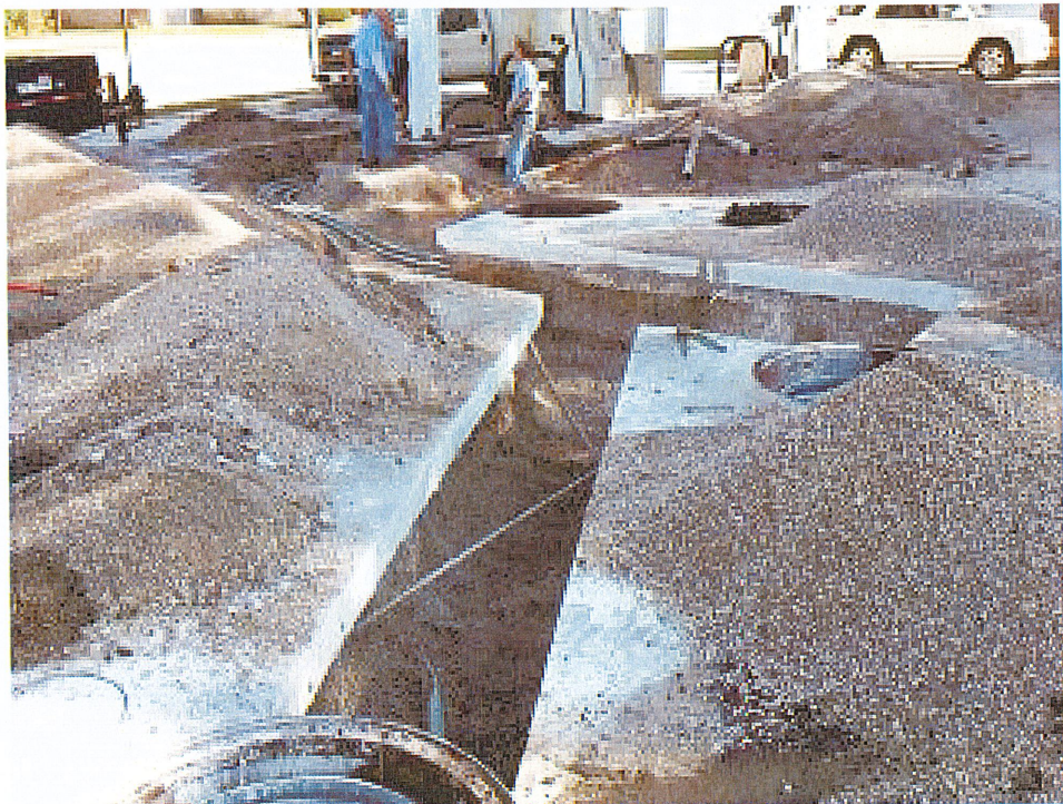
Sample location #2 collected adjacent to pump island at 3 feet below ground surface.
