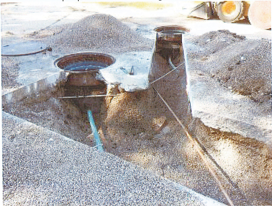
Sample point #3 collected at concurrence of piping network with underground storage tanks.
