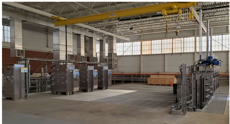
New Trojan UV Disinfection System – MMSD.
