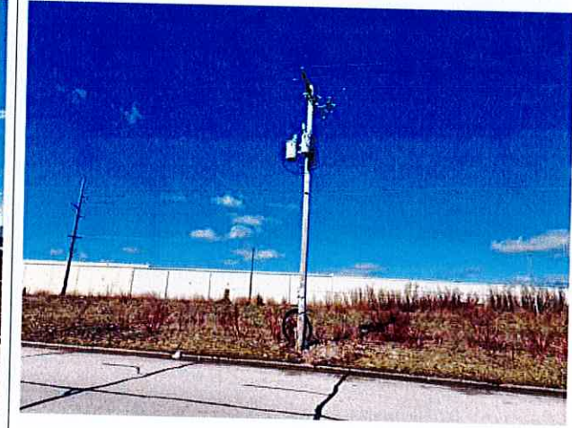
EXISTING POWER POLE / TRANSFORMER ③ SCALE: NTS
