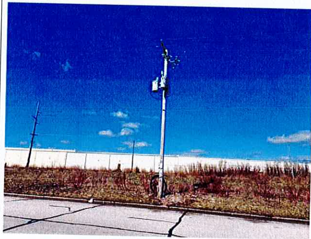
EXISTING POWER POLE / TRANSFORMER ③ SCALE: NTS
