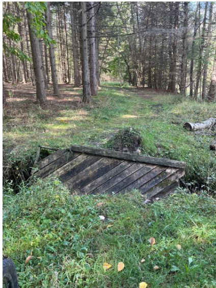
Bridge in disrepair; trail should be decommissioned.
