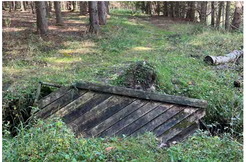
Damaged and downed bridges were documented as part of the assessment process.
