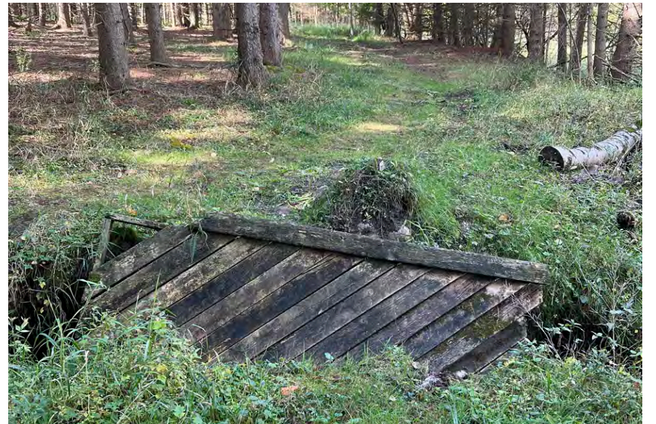
Damaged and downed bridges were documented as part of the assessment process.
