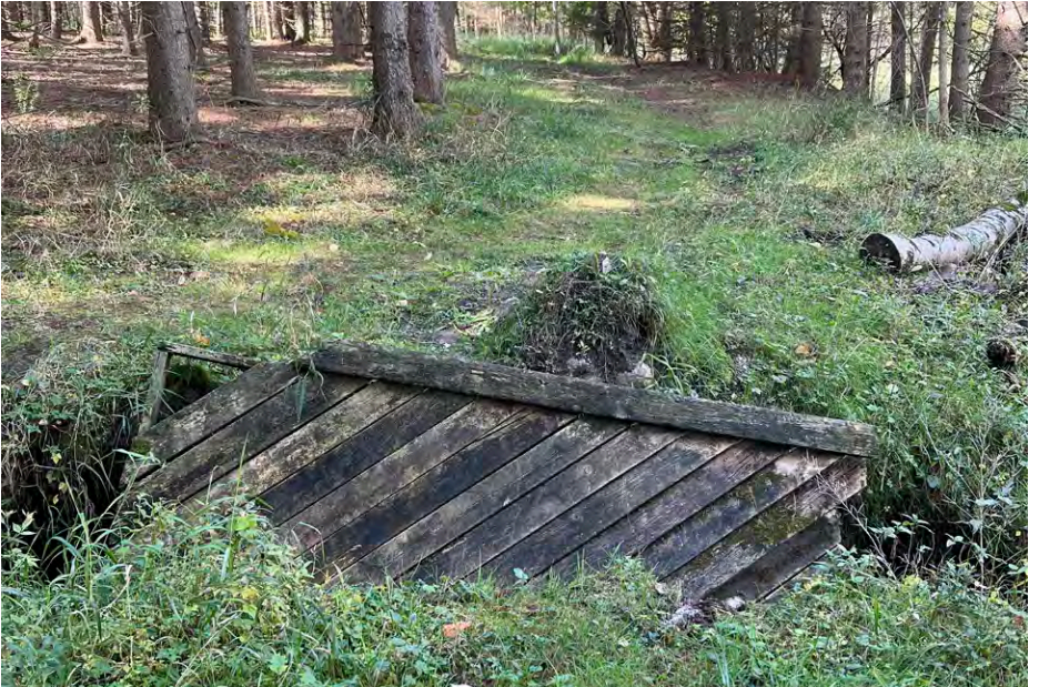
Damaged and downed bridges were documented as part of the assessment process.
