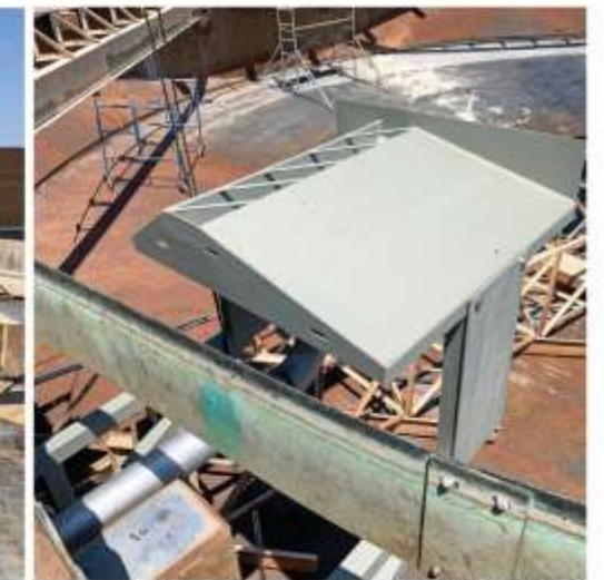
New scum box installed on Primary Clarifier #4
