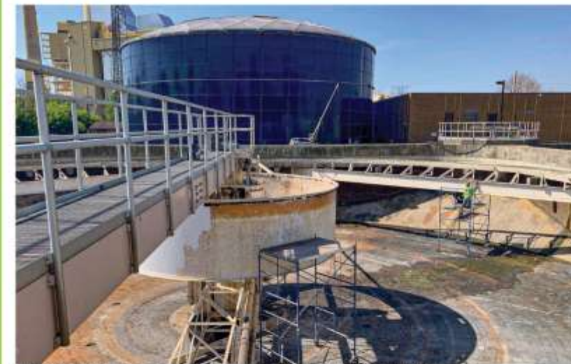
Touch up painting in Final Clarifier #2, showing corrosion on the stilling well
