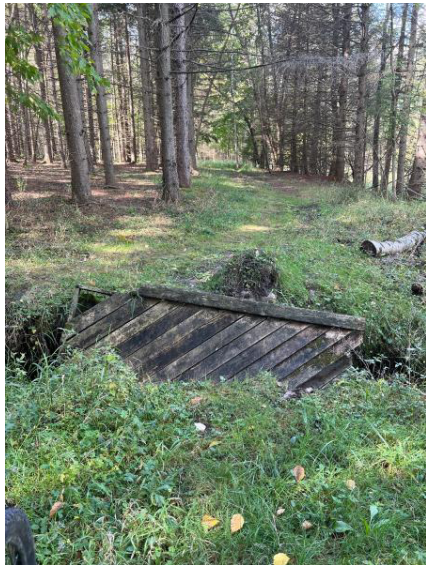
Bridge in disrepair; trail should be decommissioned.
