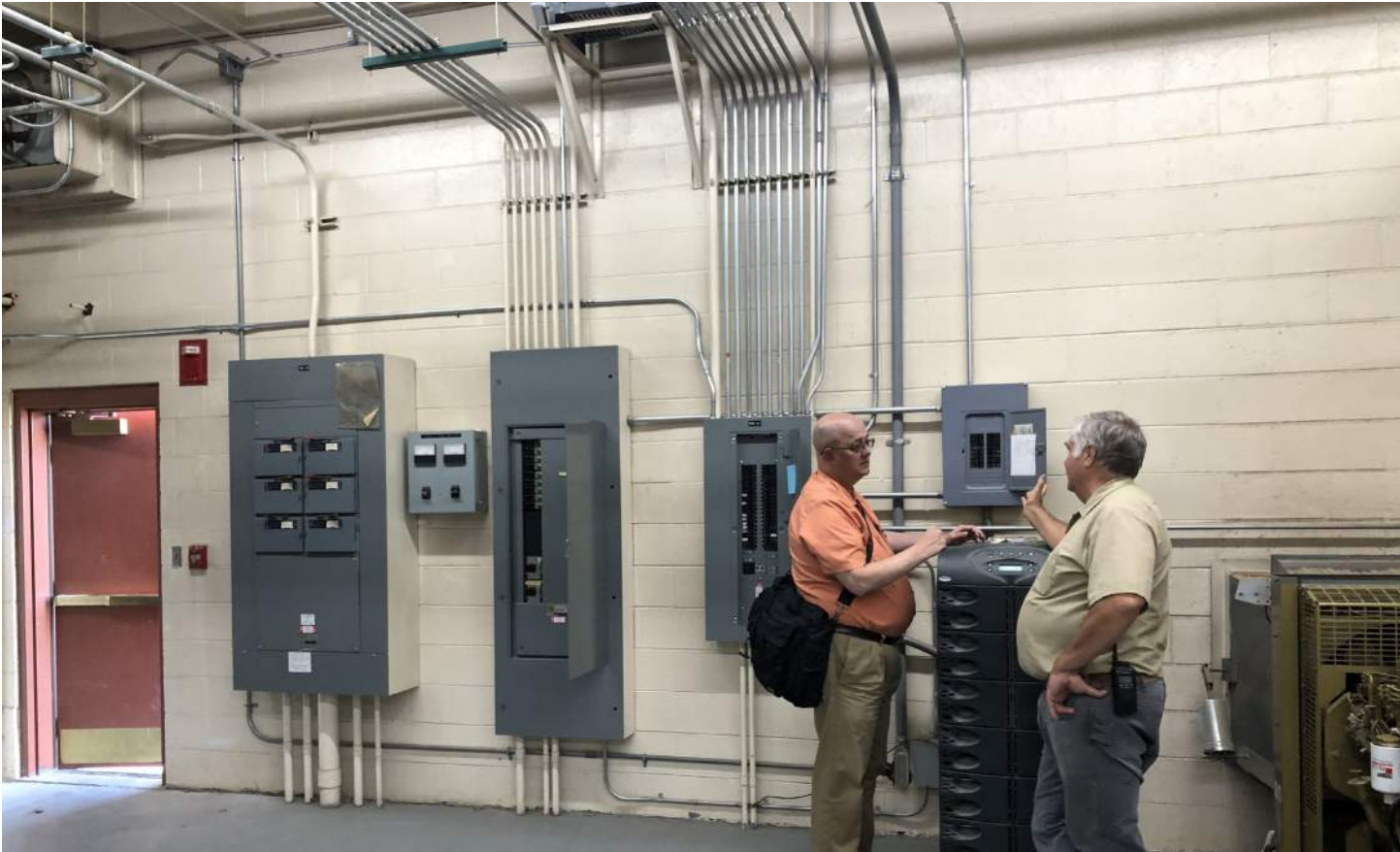
above: the majority of the electrical equipment and controls are located in the mechanical room on the lower level
