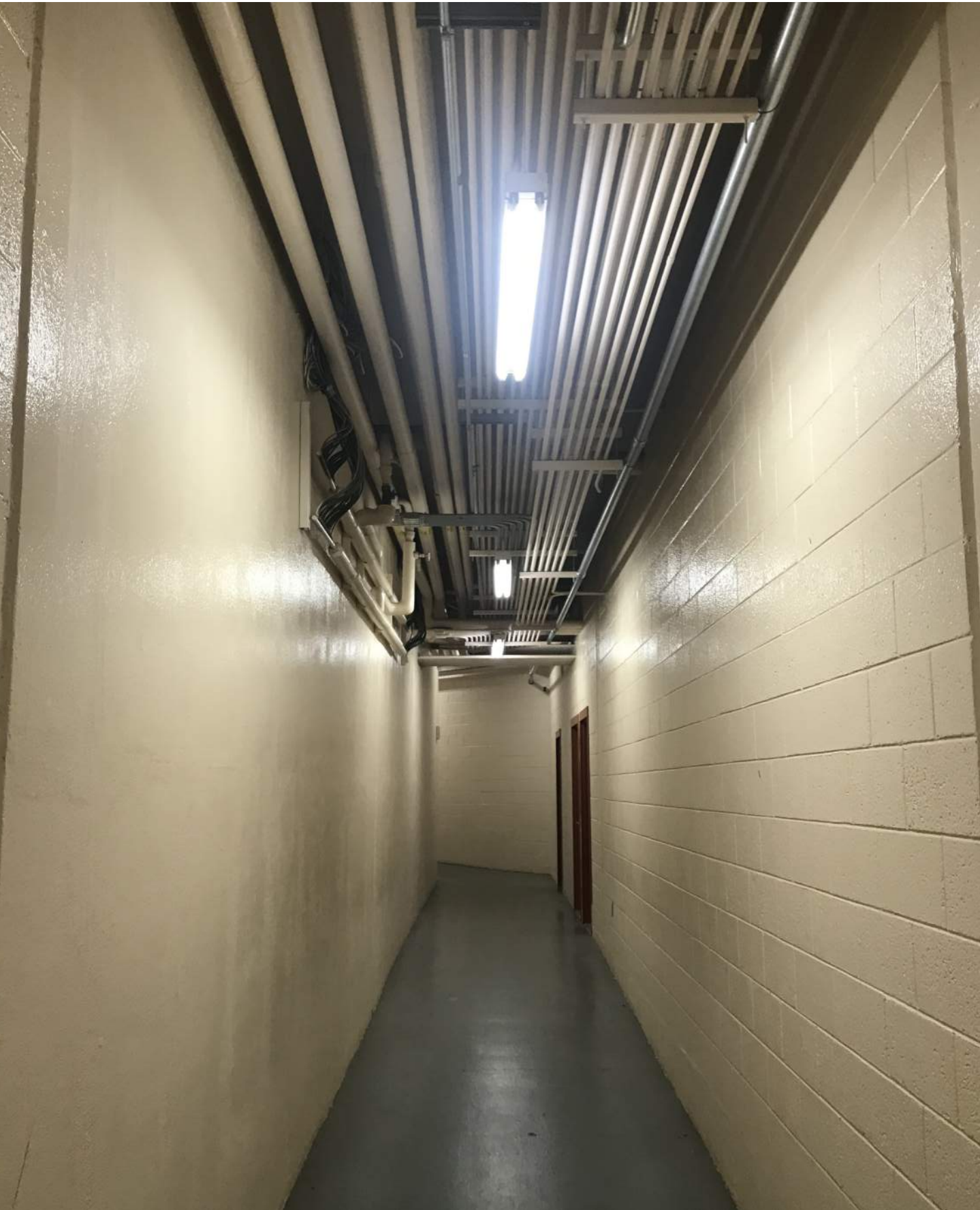
above: passage way currently used for a wide array of mechanical, plumbing, and electrical systems, located on lower level
