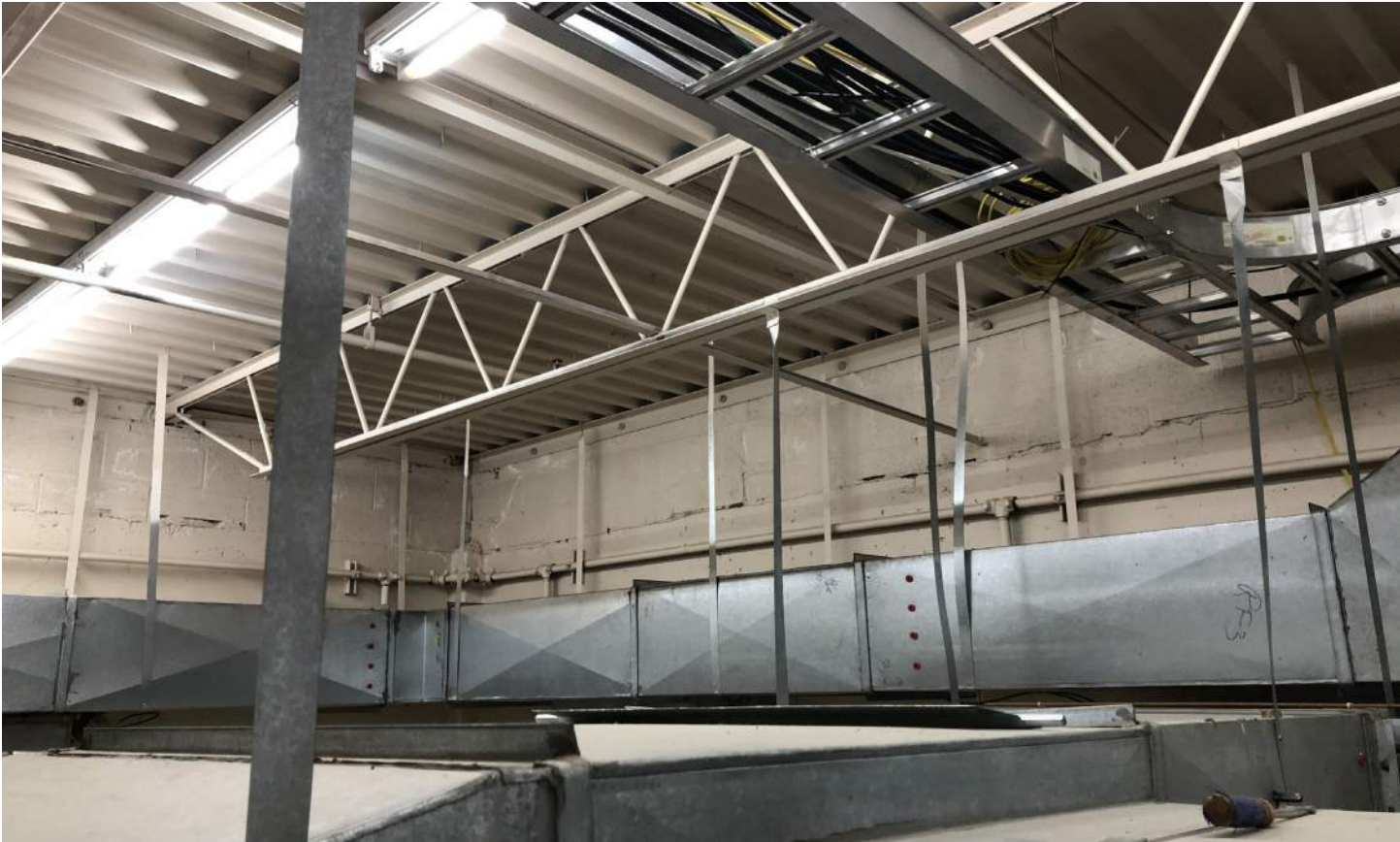
top: rooftop mechanical equipment directly above police quarters bottom: view of upper level mechanical room
