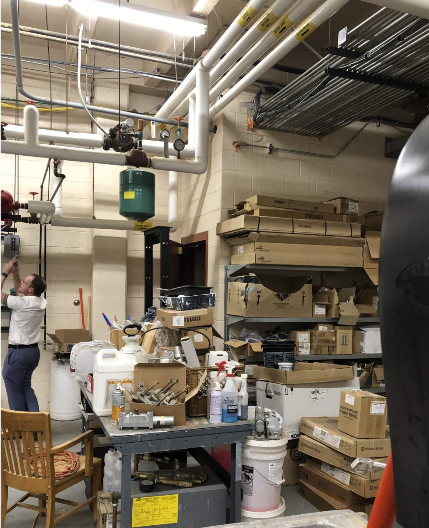
above: mechanical room view 3
