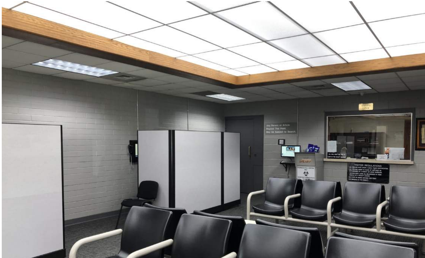
above: fluorescent lighting in the lobby (two views above), electrical engineer proposes LEDs throughout the facility only where renovation is taking place, see bullet "10"
