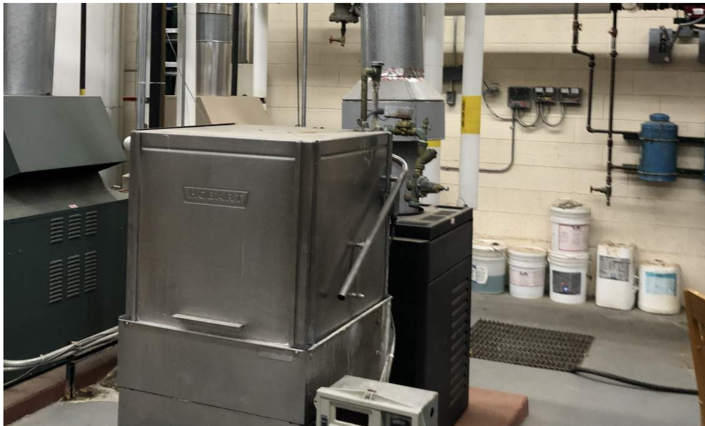
top: mechanical room view 1 bottom: mechanical room view 2
