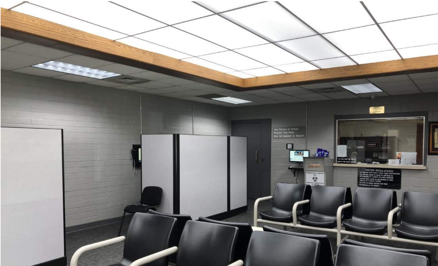
above: fluorescent lighting in the lobby (two views above), electrical engineer proposes LEDs throughout the facility only where renovation is taking place, see bullet "10"
