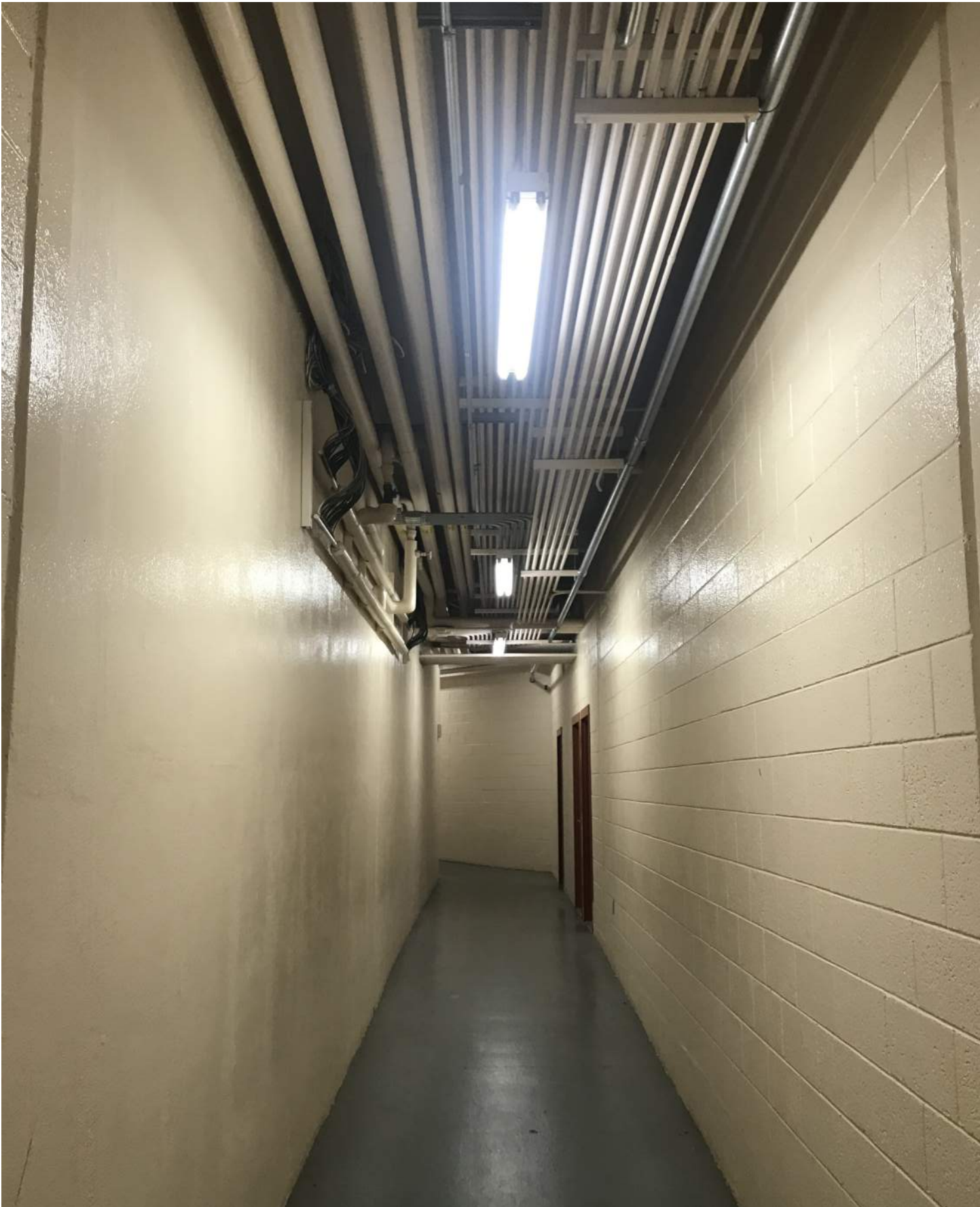
above: passage way currently used for a wide array of mechanical, plumbing, and electrical systems, located on lower level
