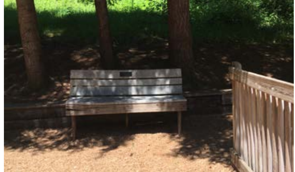
3. Park seating options are deteriorating, with wood rot and sinking planks
