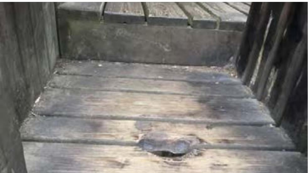
4. Decaying, splitting, and rotting decking causing tripping hazards
