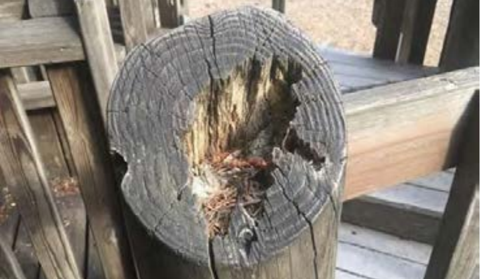
1. Splintering and declining wood frame
