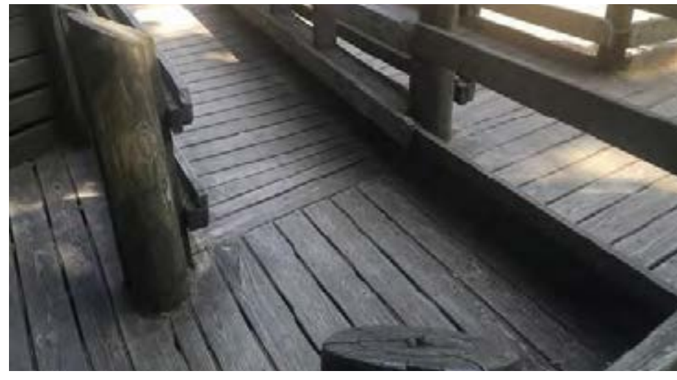
6. The current ADA accessible path is deteriorating, with visible signs of splitting and rot
