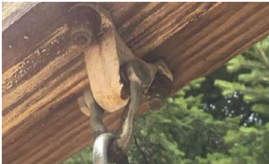
5. The swing hangers are showing wear and rust
