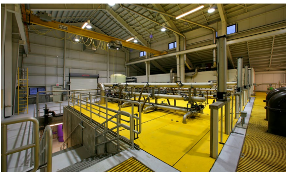
NLRSD WWTP Membrane Tanks
