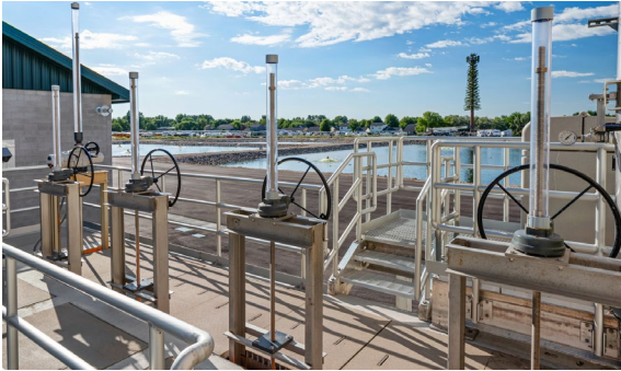
SSWD WWTP MBR Splitter Box
