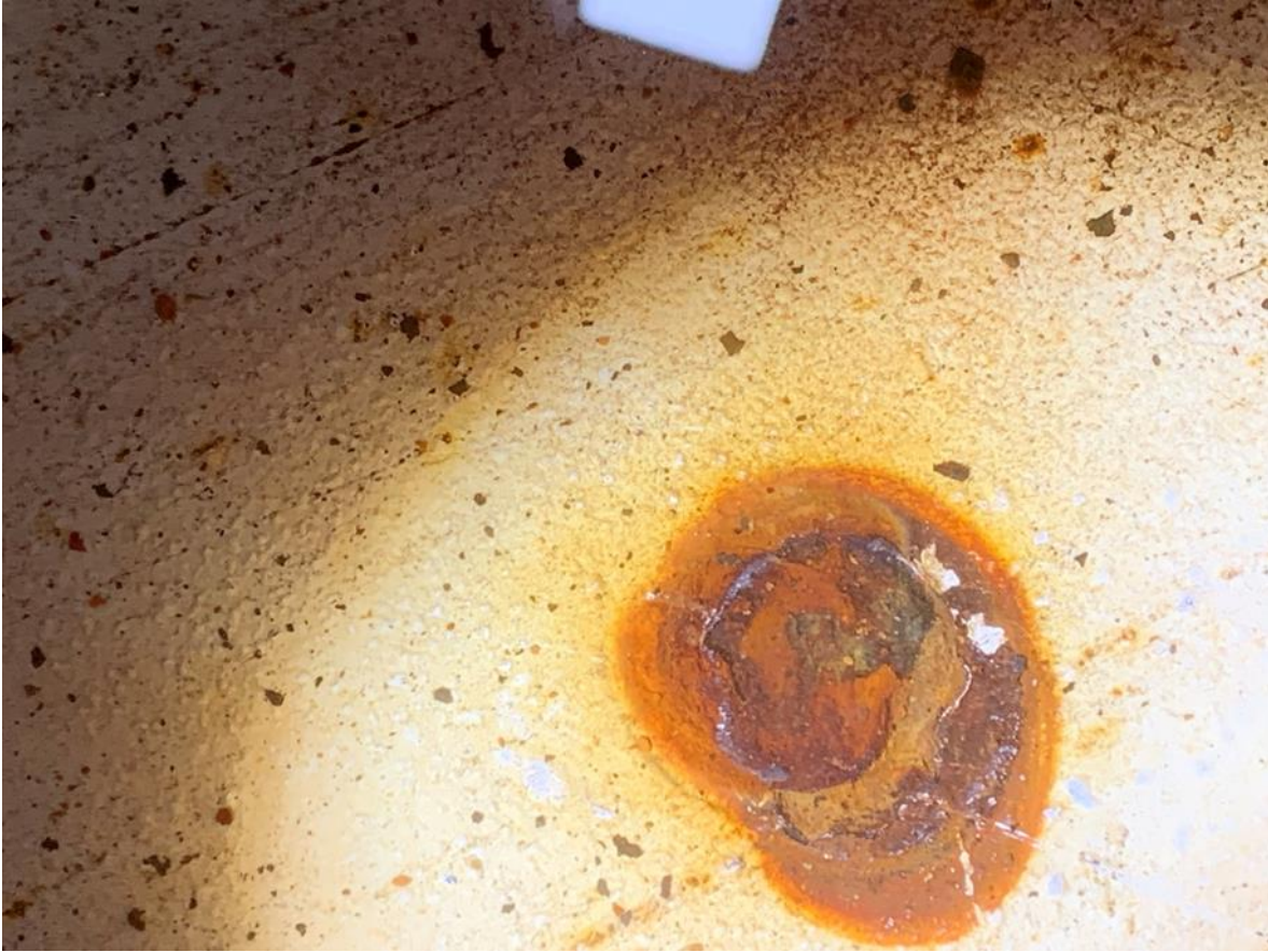
FIGURE 4 - TANK FLOOR PITTING
