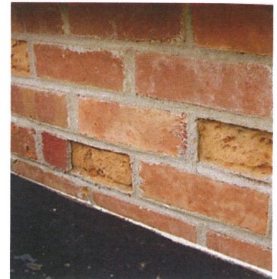
[2] Not Recommended: The use of inappropriate Portland cement mortar to repoint these soft 19th-century bricks has caused some of them to spall. Photo: Courtesy Nebraska State Historic Preservation Office.
