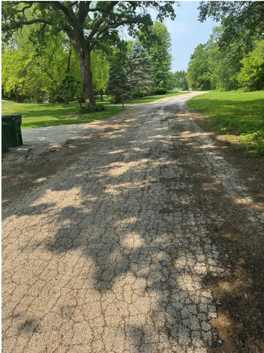
Windflower Way | Poor condition
