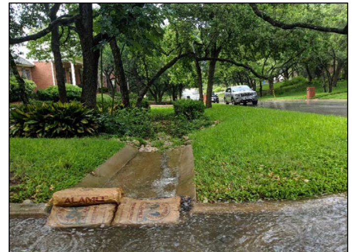
200 Wallis Drive, during rain event. 06/06/2019
