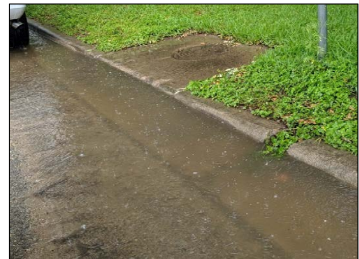
Pond inlet during rain event. 06/06/2019
