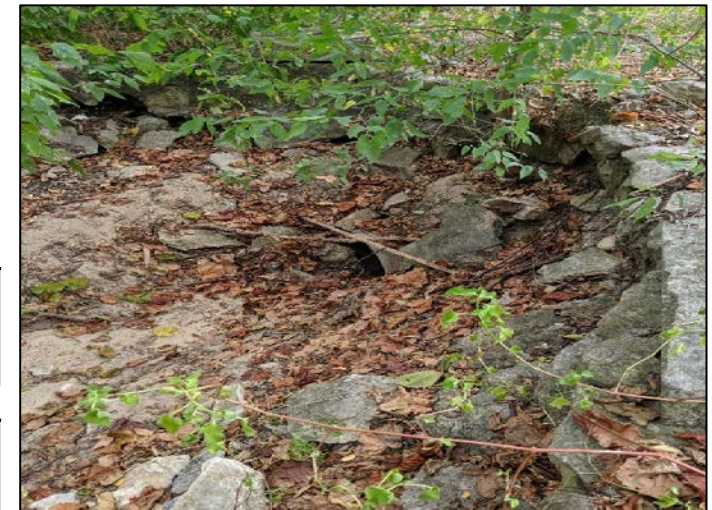
Half buried culvert at Rollingwood Drive. 09/11/2019
