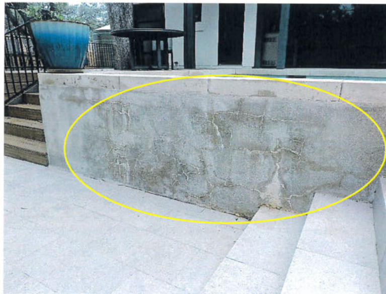
Figure 4: Cracking distress and efflorescence of exterior spa wall
