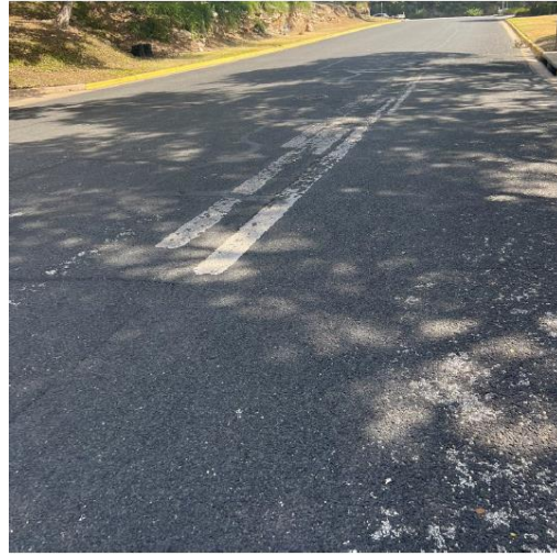
Beecave Woods Dr PCI Rating = 80 Good Strategy: Crack sealing, rejuvenators, fog sealing, pothole repairs
