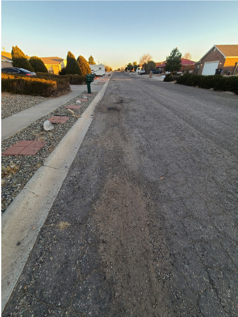
Figure 2: Excessive cracking and subgrade exposure
