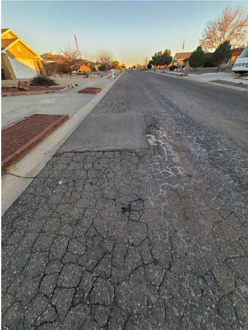
Figure 4: Alligator cracking and subgrade failure
