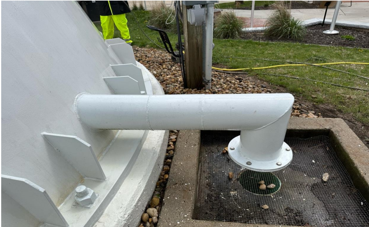
Base Cone After Power Washing
