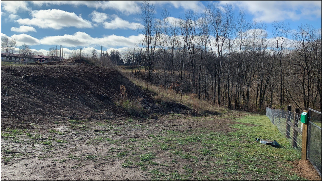
Figure 7. Area of the retaining wall adjacent to the dog park, view southwest. Note the slope and large historic fill pile. Photo taken 11/11/22.
