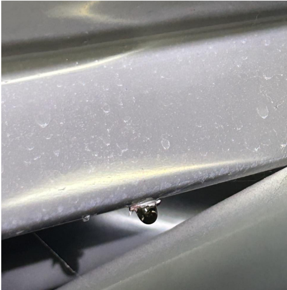
ABOVE THE MECHANICAL BOX IN HALLWAY ACROSS FROM THE LIBRARY
