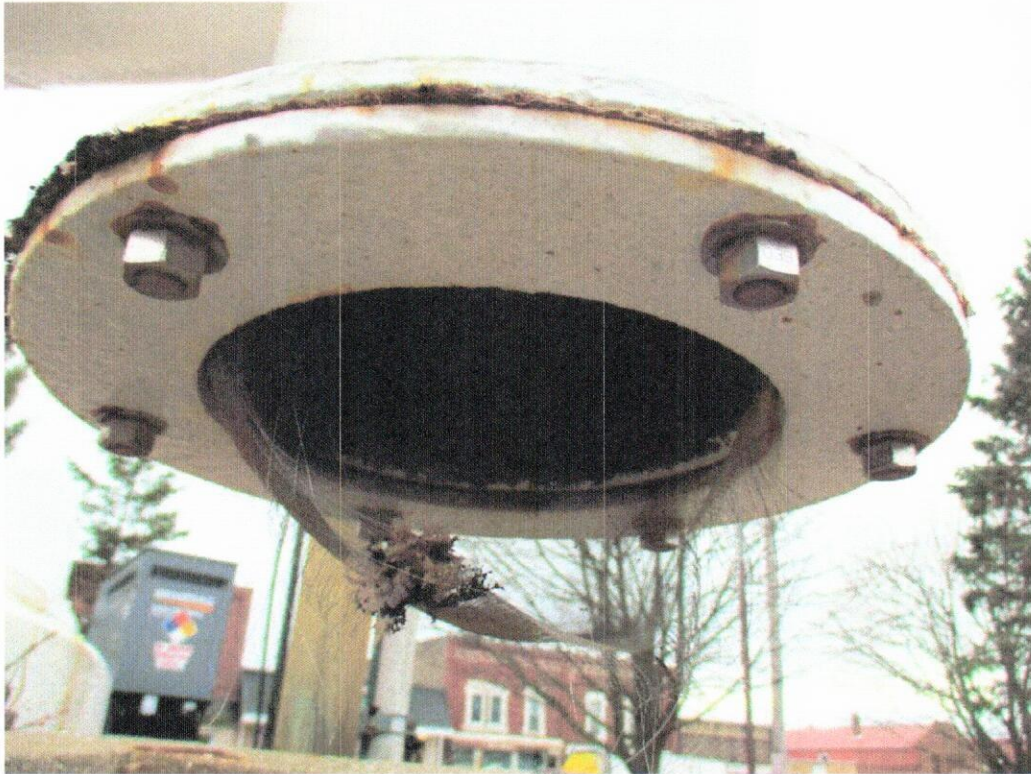
Exterior Overflow – Poor Condition – Broken Mesh
