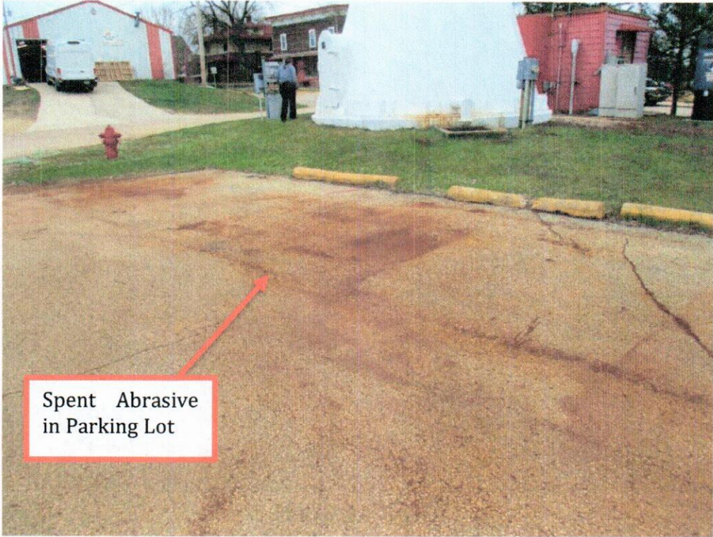
Site Parking Lot - Residual Spent Abrasive
