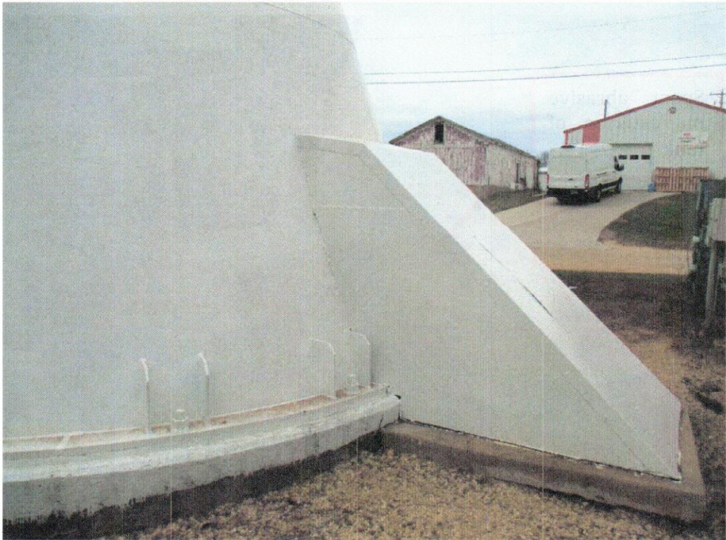
Exterior Base Bell - Gap in Telecom Structure
