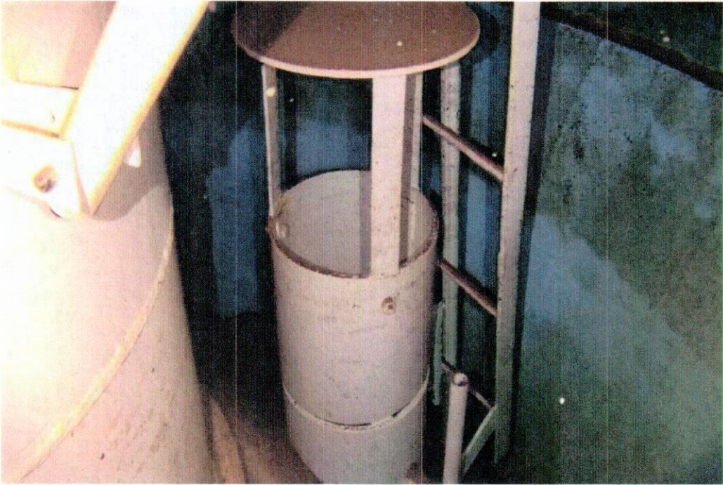
Interior Wet Fill Pipe & Deflector Plate- Good Condition
