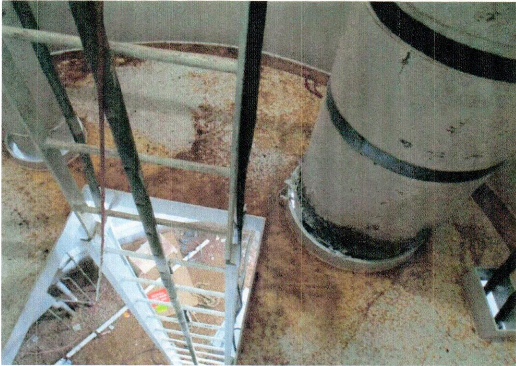
Condensate Platform - Fair Condition - Debris & Staining
