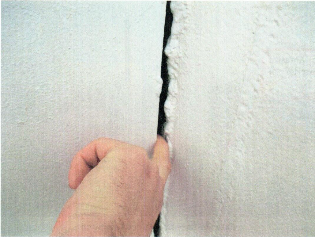
Exterior Base Bell - Gap in Telecom Structure
