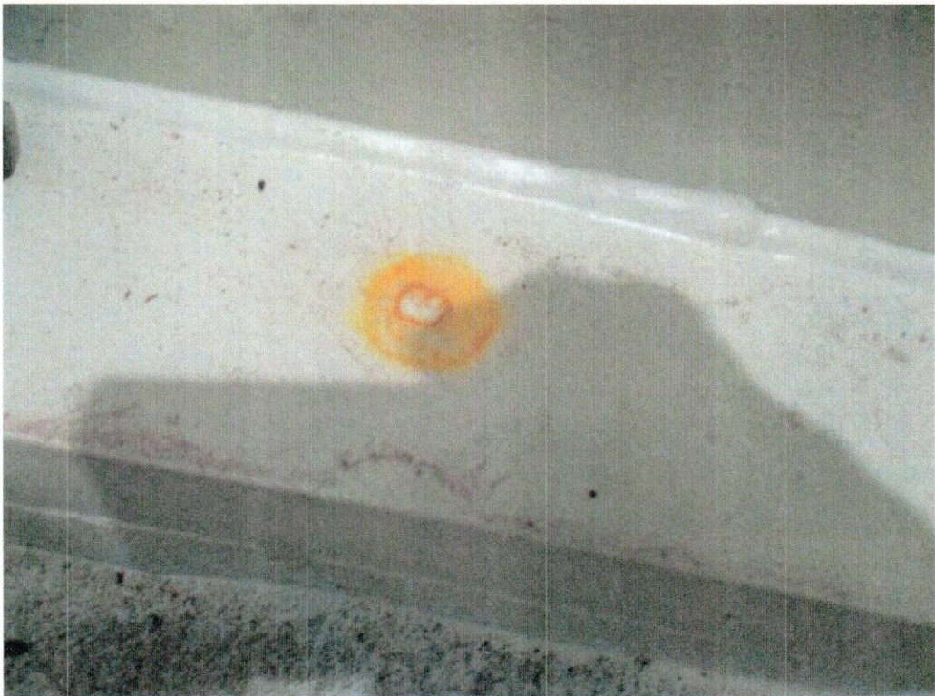
Interior Dry Base Bell - Good Condition - Washer Stain
