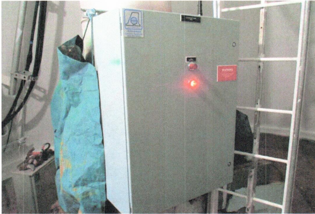
Scada Fill Panel - Good Condition
