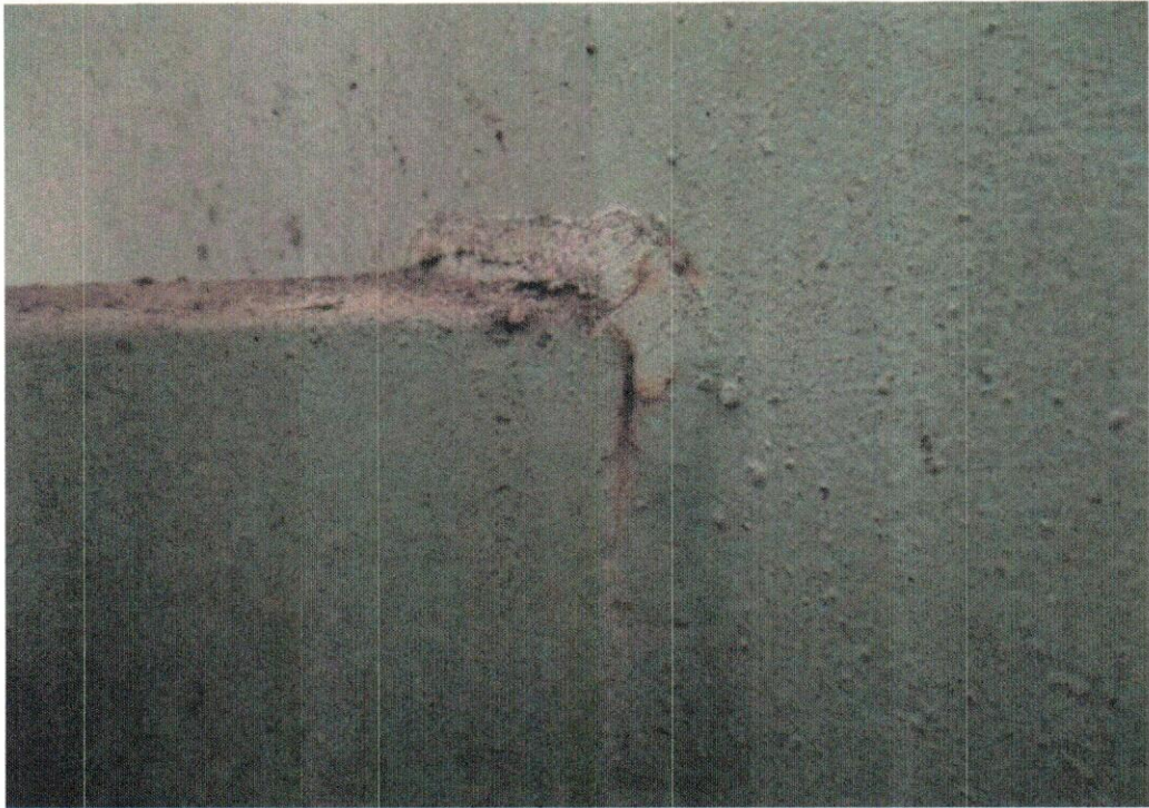
Riser - Coating Crack
