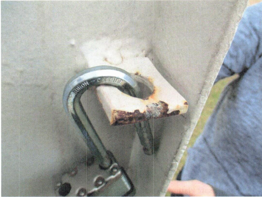
Tank Lock - Good Condition
