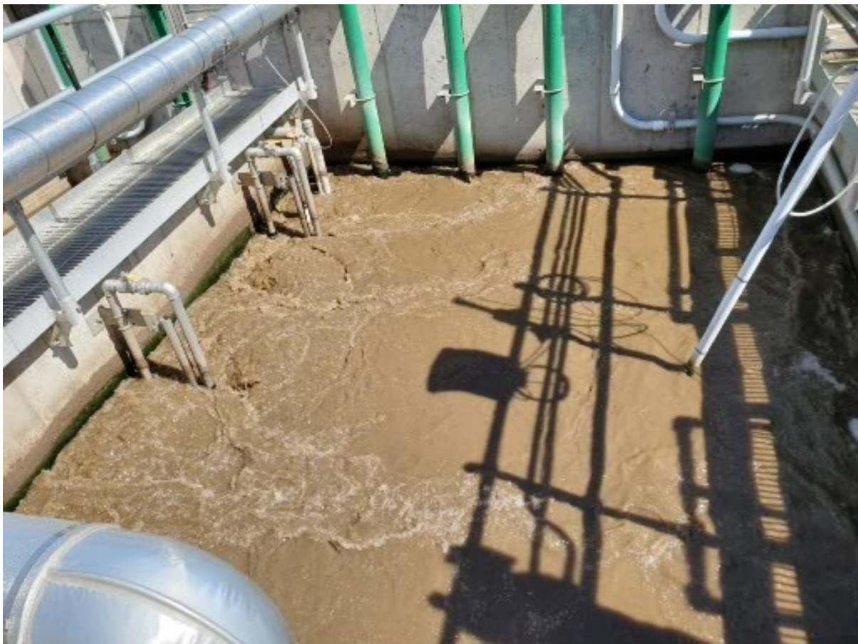
Picture #2 - Aeration Basin in Fill/Aeration Mode
