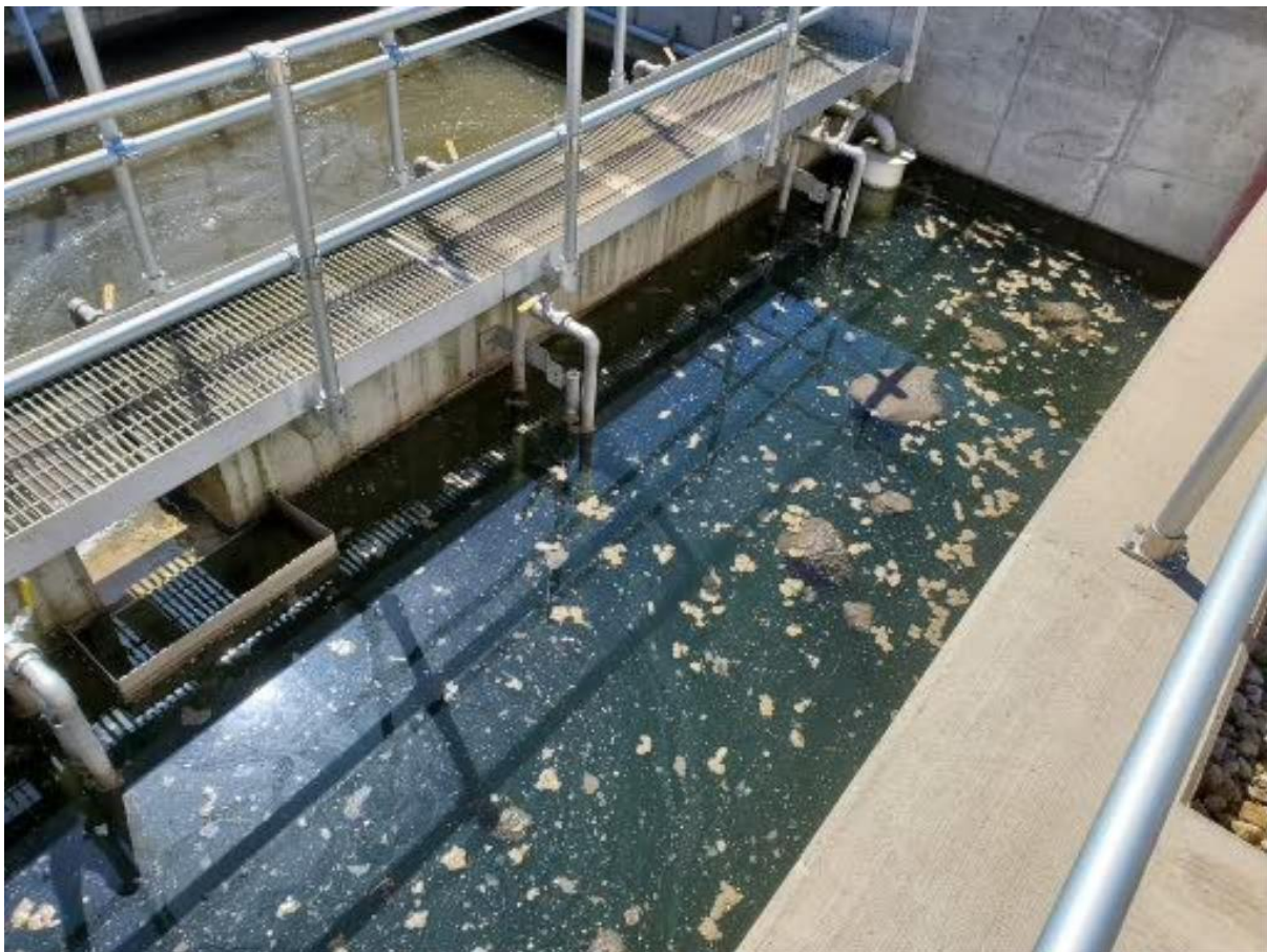
Picture #4 - Aeration Basin in Anoxic Zone
