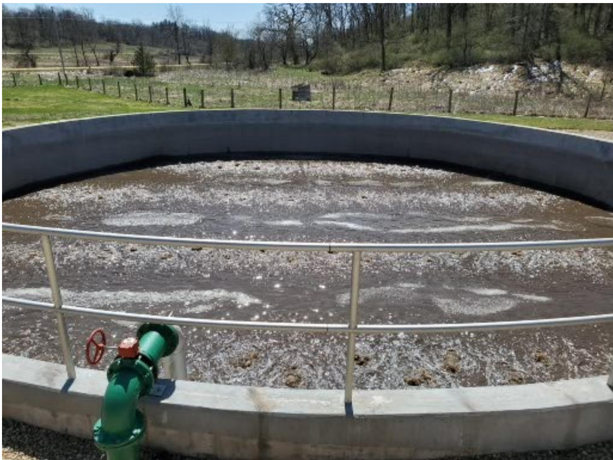
Picture #6 - Aerated Sludge Storage
