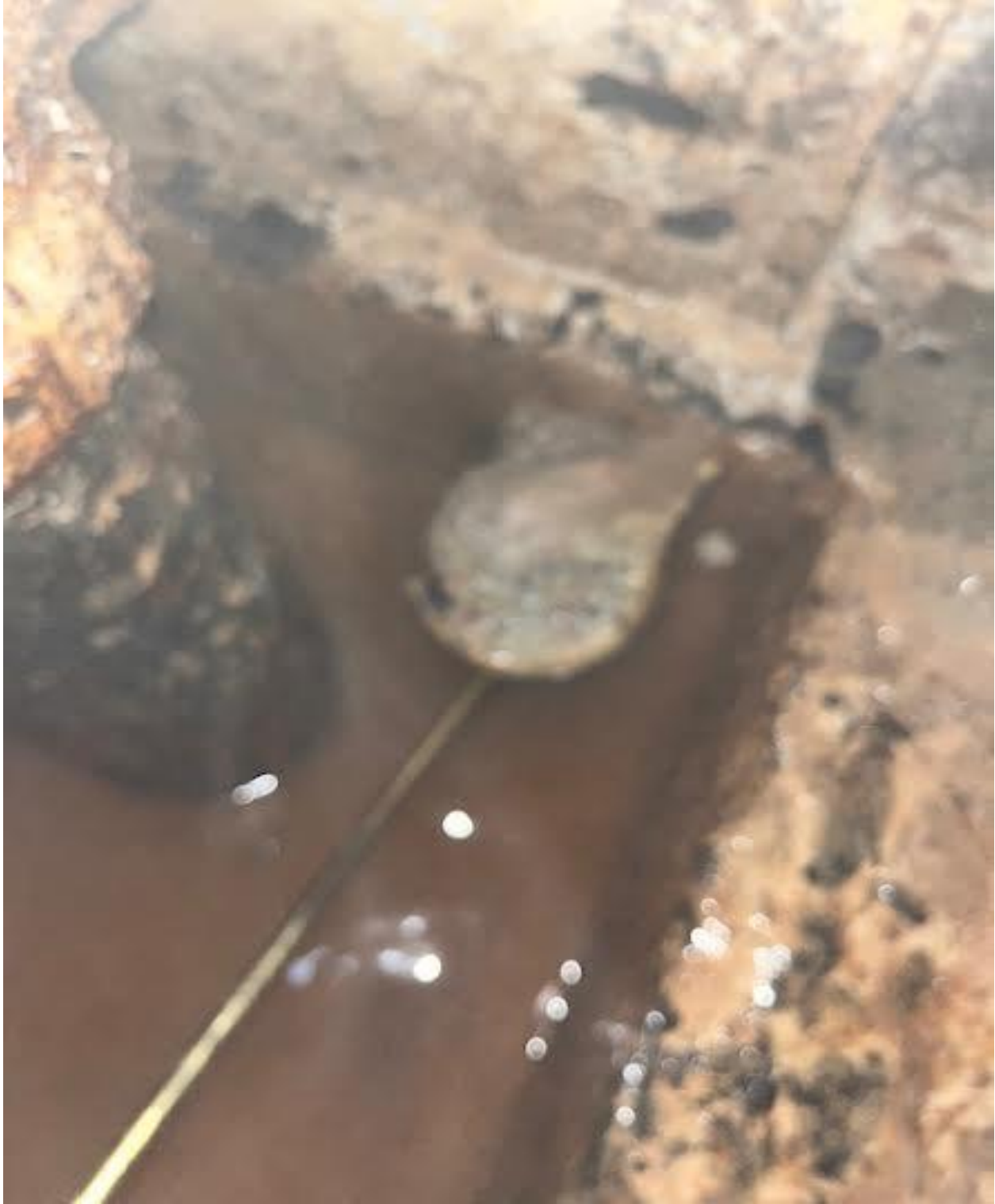
The Sump was Filled with Sediment
