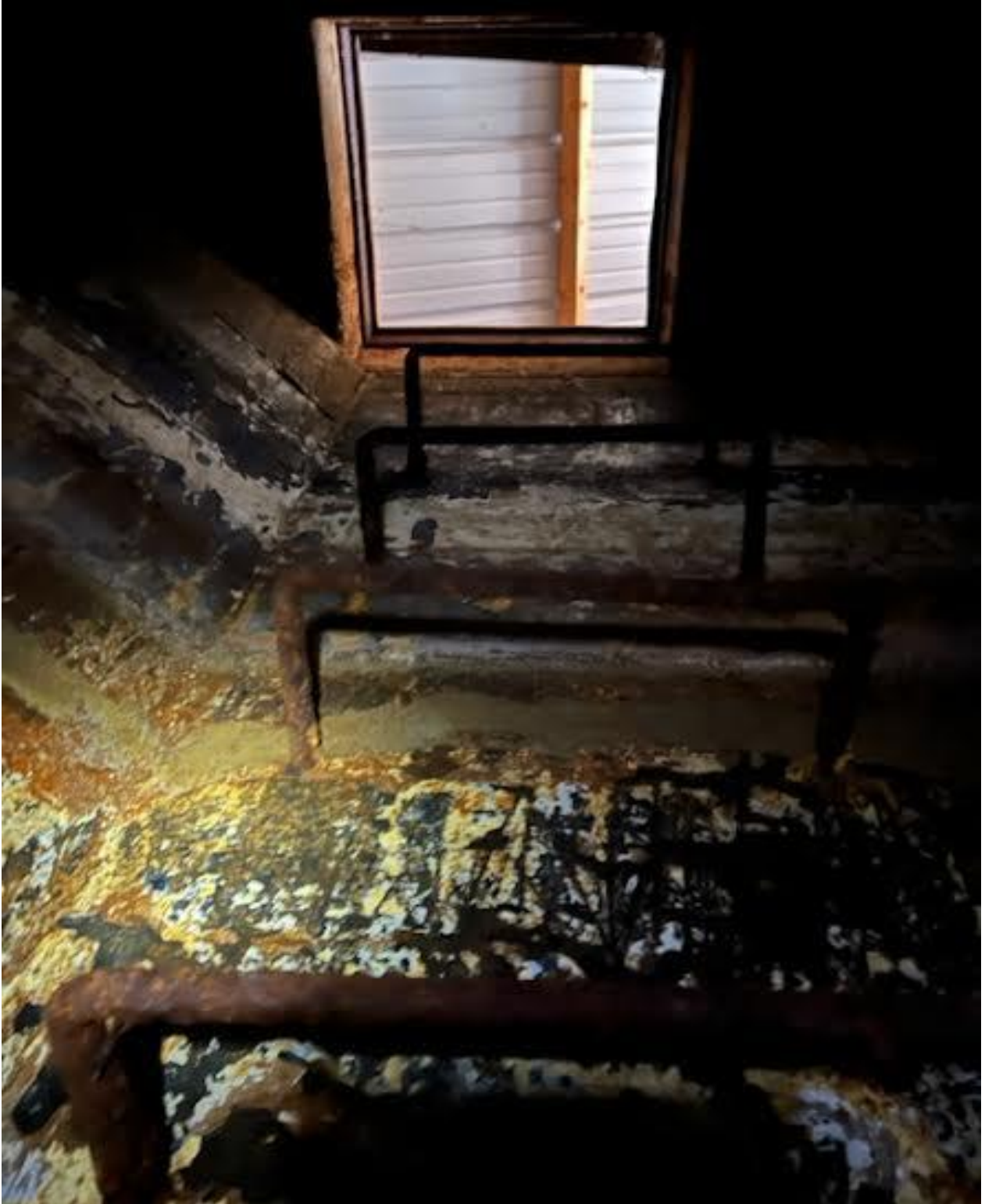
The Metal Ladder at the Northwest is in Poor Condition
