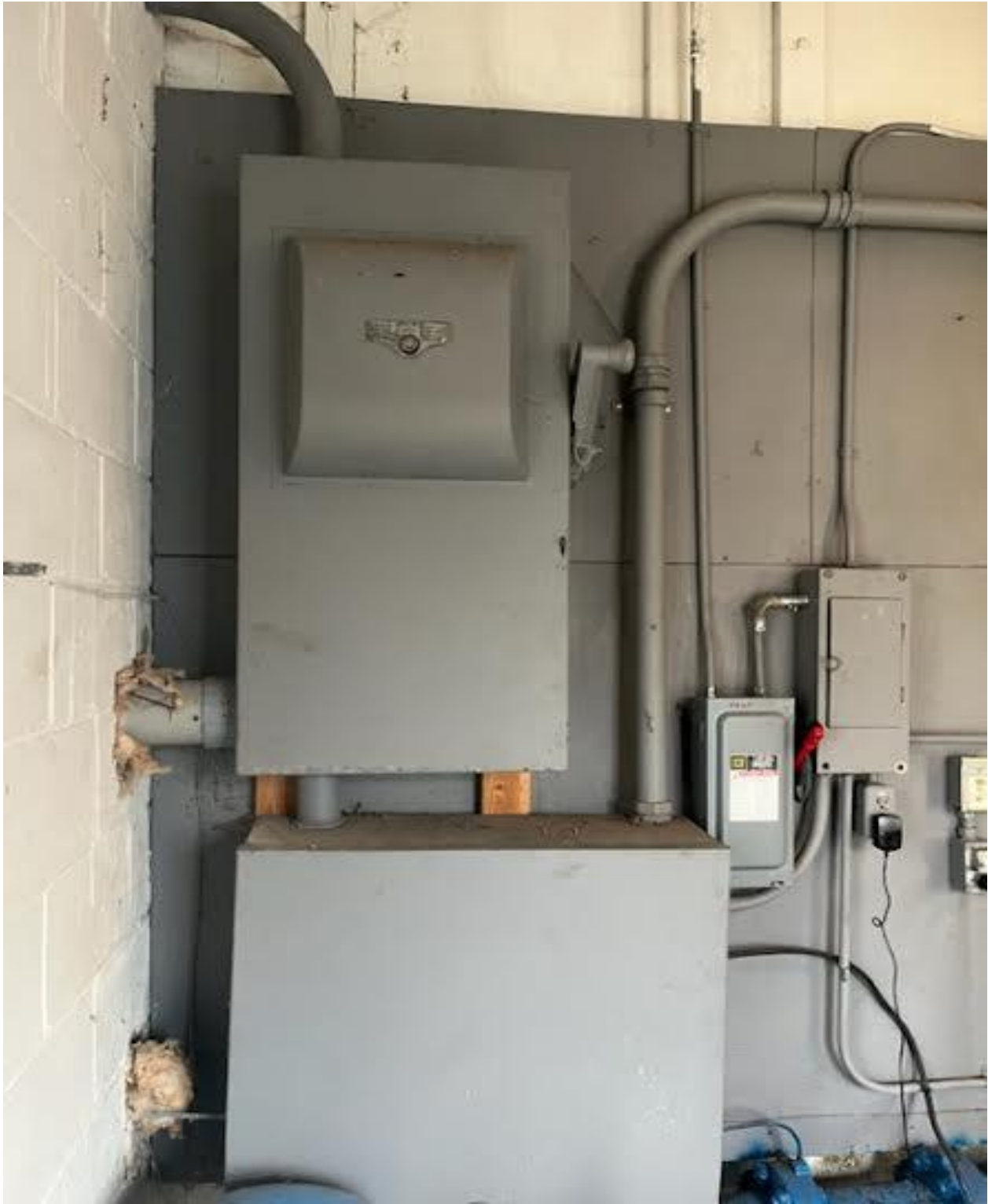
The Electrical System Is in Good Condition
