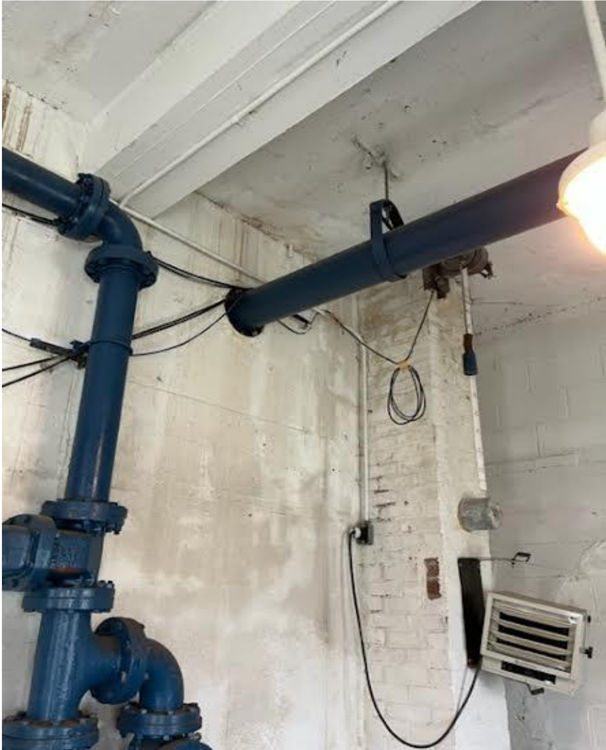
Overflow Pipe is in Good Condition
