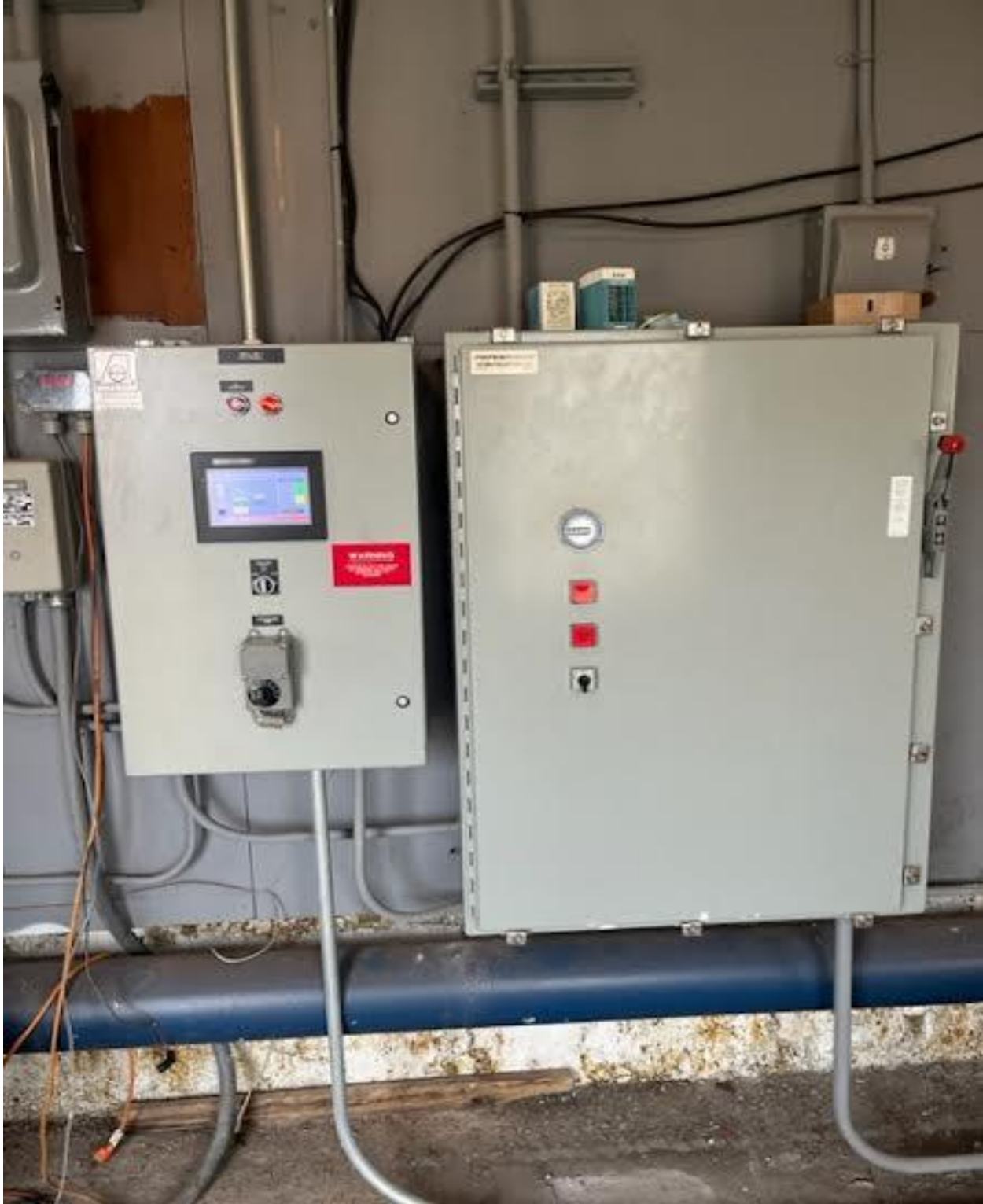
The Electrical and Fill Telemetry
