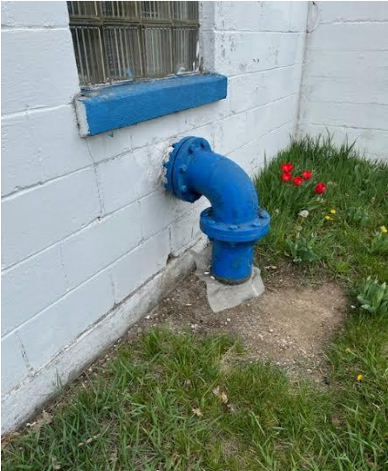
Overflow Pipe is in Good Condition
