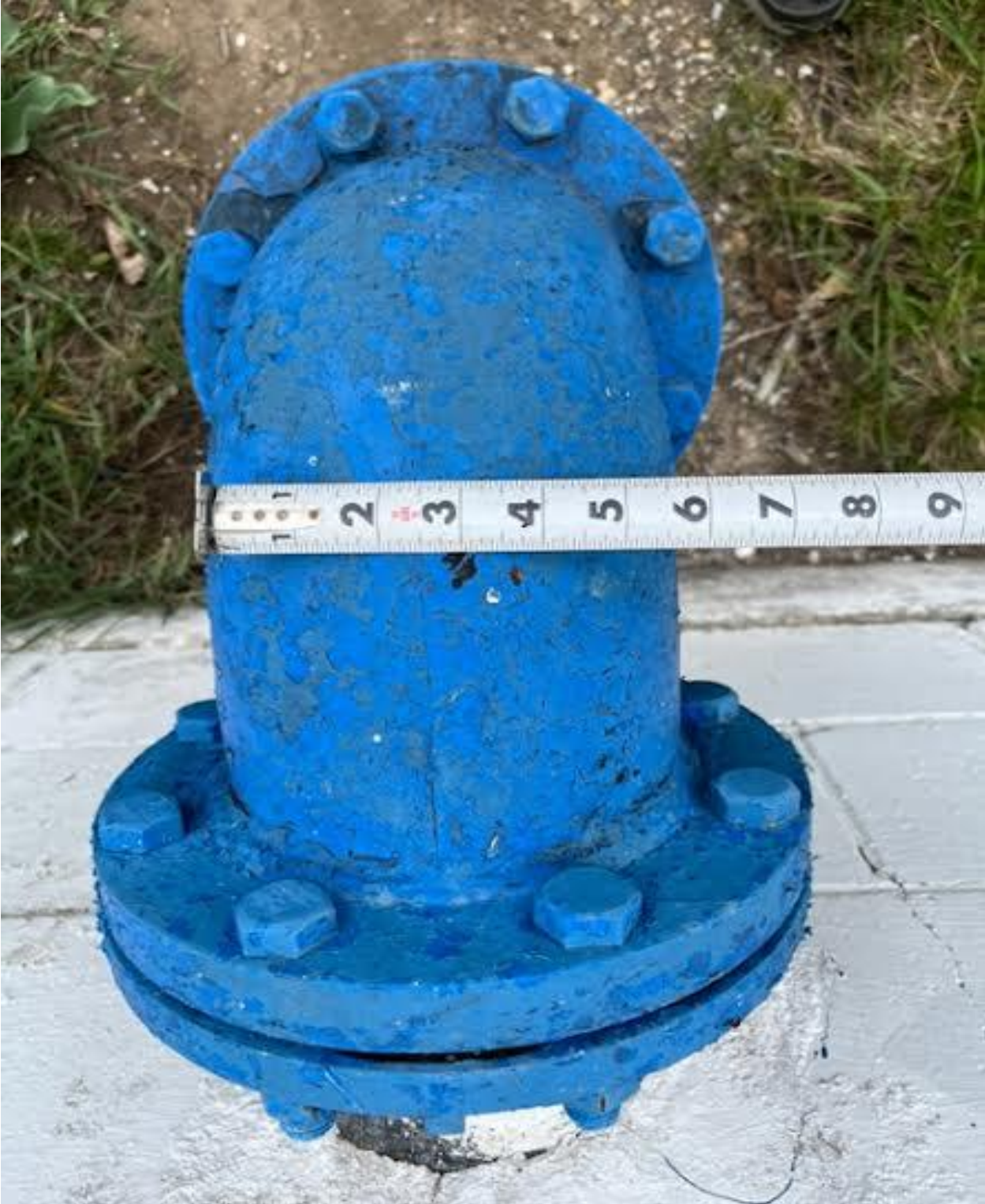
6" Overflow Pipe is in Good Condition
