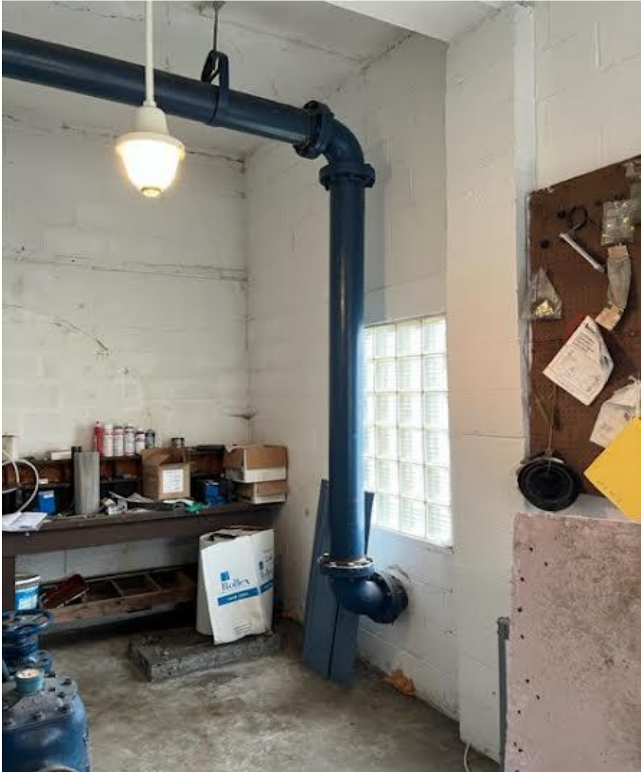
Overflow Pipe is in Good Condition
