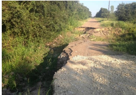
Road condition after significant flooding from FEMA Disaster DR-4272.
