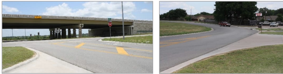
Left: Widening and realignment of intersection with US 290 Frontage Road. Right: Widening and realignment of Stringer Street.
