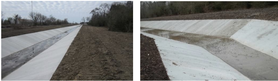
Views of the completed reinforced concrete slope paving in an existing drainage channel.
