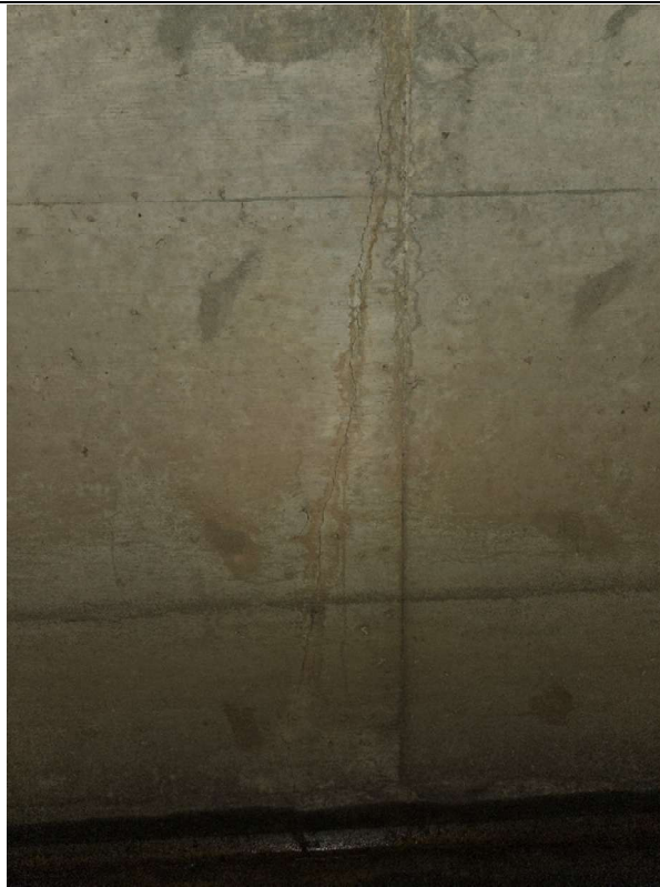
Photograph: 40 | Photo of cracks in concrete channel.
