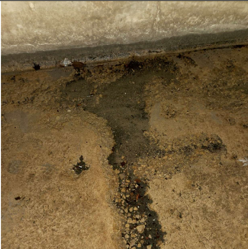
Photograph: 38 | Spalled concrete within channel concrete floor.
