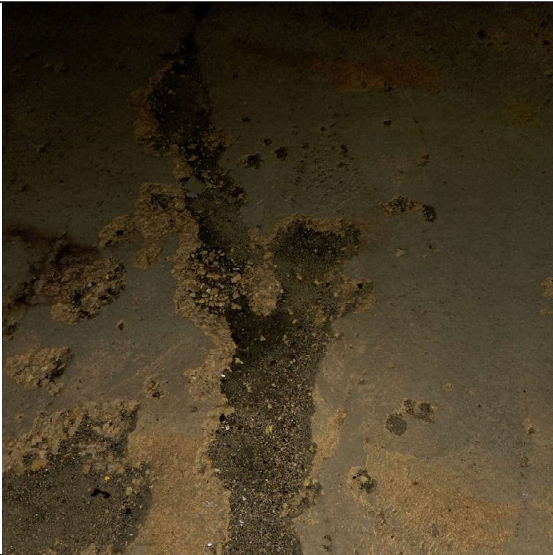
Photograph: 37 | Spalled concrete within channel concrete floor.
