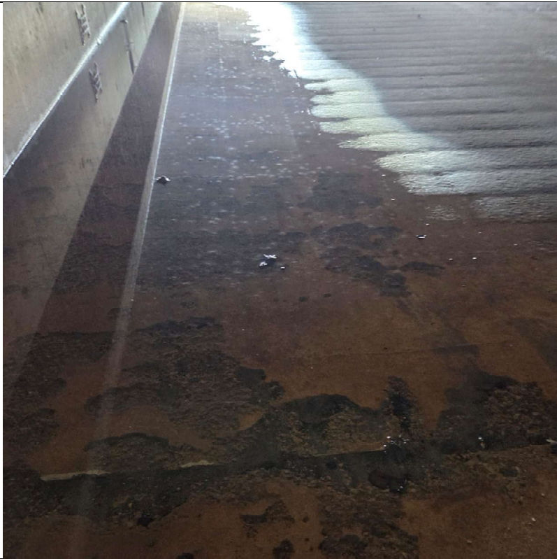
Photograph: 35 | Photo of spalled concrete within channel concrete floor.
