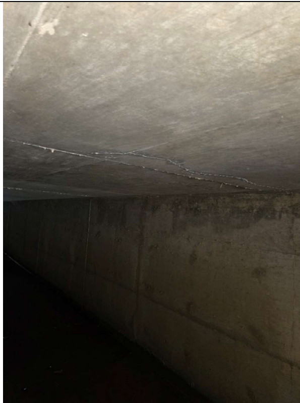
Photograph: 42 | Photo of crack in concrete channel.
