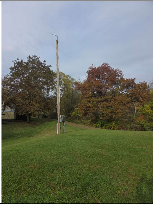
Photograph: 7 | Control panel in good condition.
