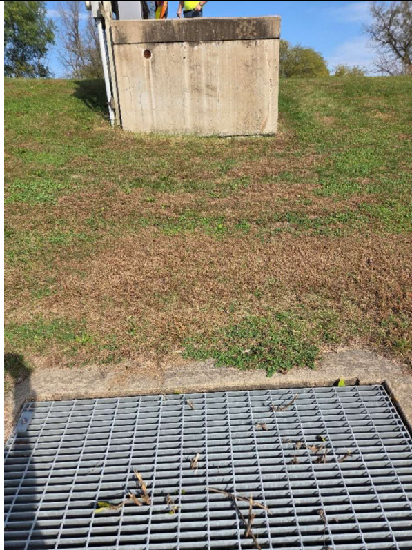
Photograph: 26 Viewing gate valve and grate at retention basin. Debris to be removed.
