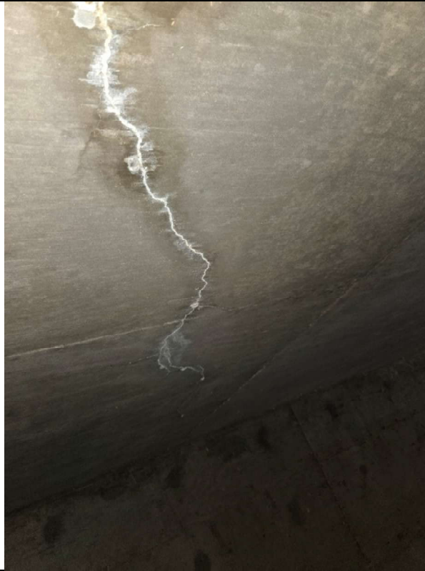
Photograph: 43 Photo of crack in concrete channel.
