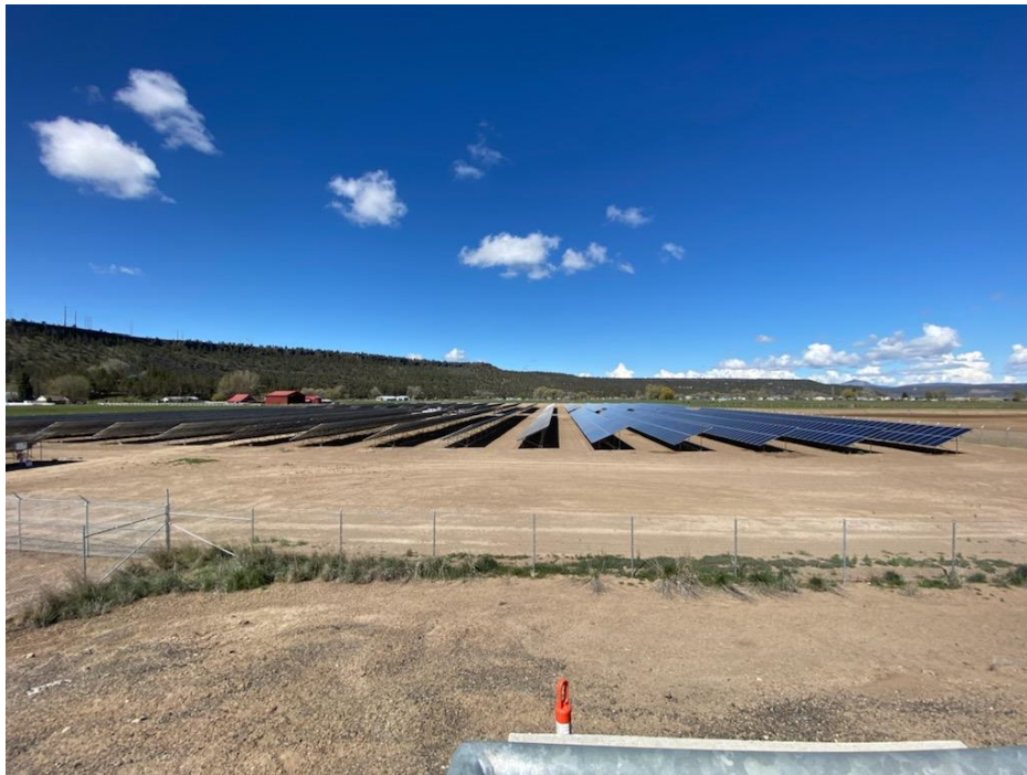
Completed fencing for the solar farm by the wastewater treatment plant. – May 2022
