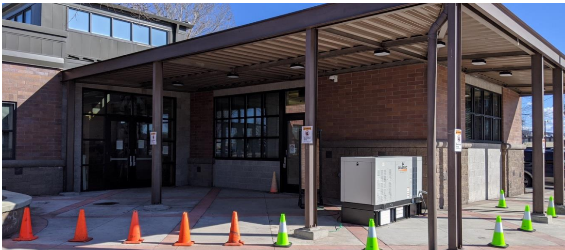
Backup generator needed for the dispatch center with the move to City Hall which was set up by IT.
