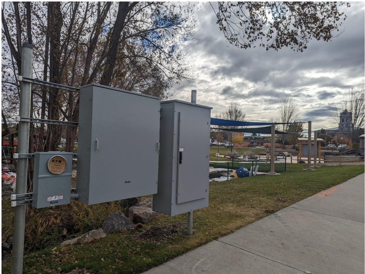
EV Charging station work was completed during the first quarter near the Kiwanis Splash Pad.
