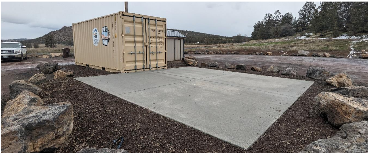
New concrete slab poured in February at the Barnes Butte Recreation Area for the use of a telescope.
