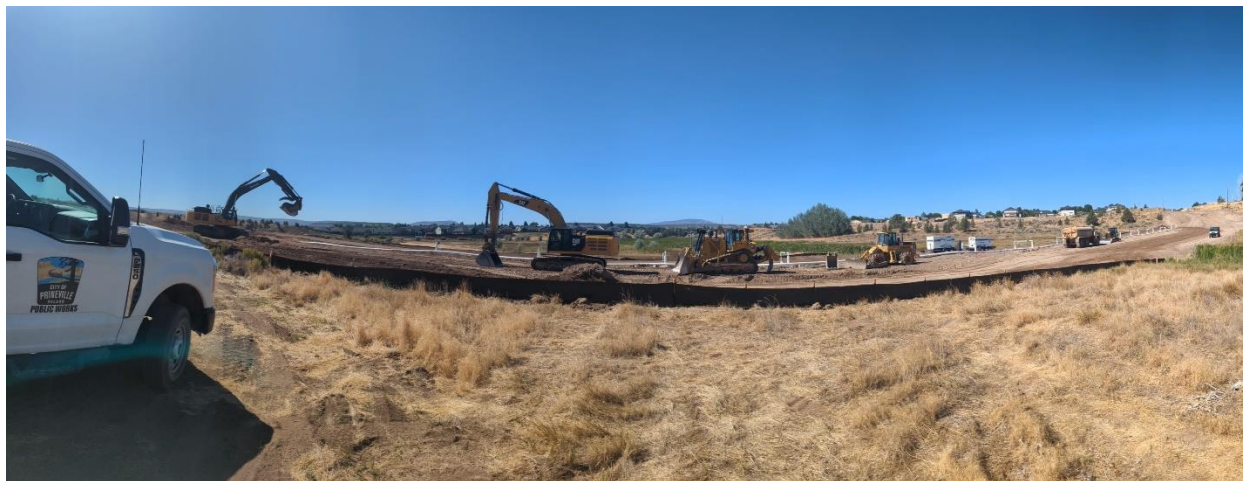
The Construction of Combs Flat to Peters Road Extension started in Q1 of FY 25.
