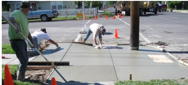
Sidewalk improvements being done improving ADA accessibility on the corner of NE Fairview and 1st Street.
