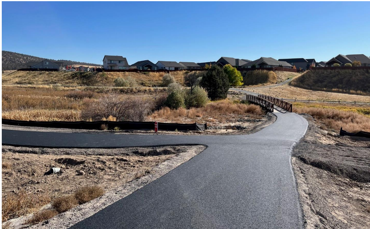
Trail paving work started at the tail end of the second quarter at Barnes Butte
