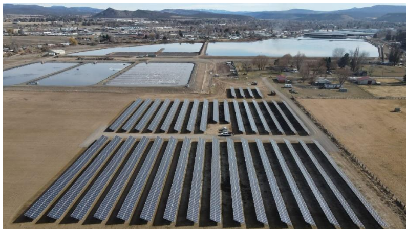
Solar field at the wastewater treatment plant facility.
