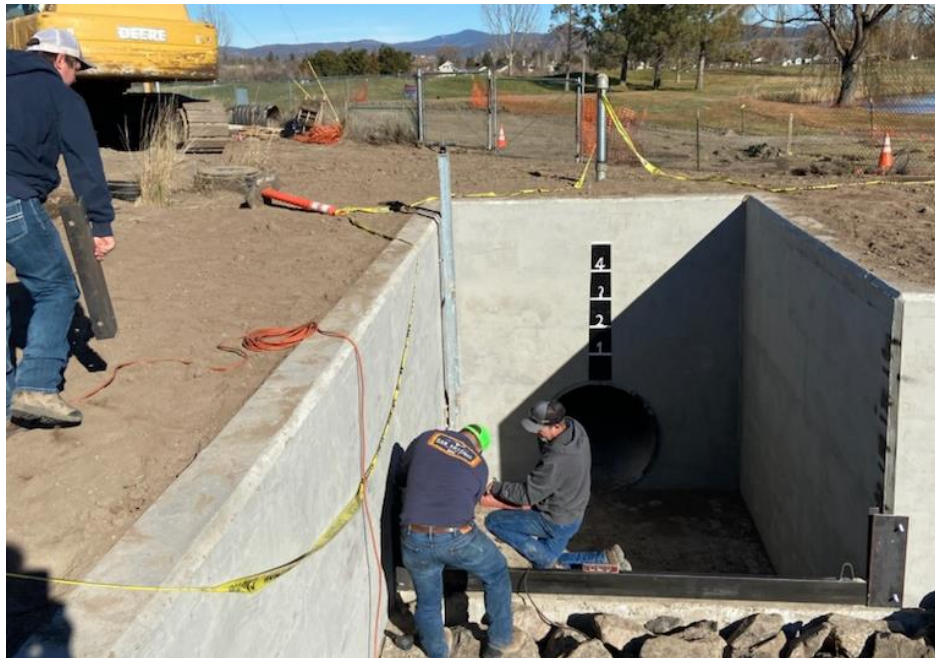
Public Works crew working on the Peoples Irrigation Ditch project in January 2022.
