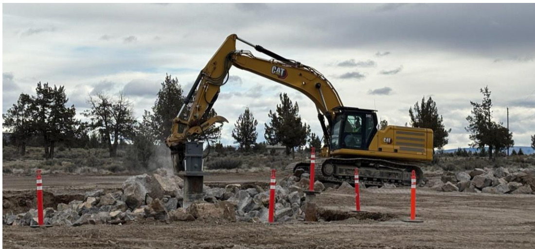
ASR well work being done during the third quarter new the airport.
