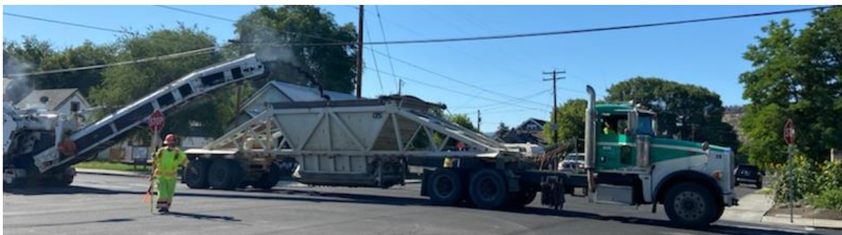
Second Street paving, part of the 2020 paving project, that took place during the first quarter.
