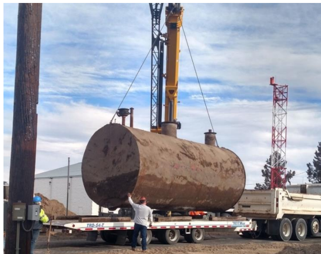
With the new system coming on line in the second quarter, the old fuel tanks were removed.
