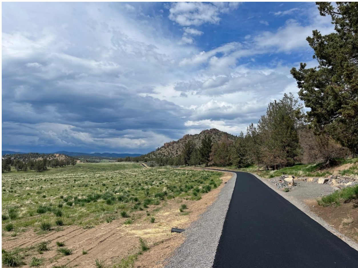
Trail paving work was completed during the fourth quarter at Barnes Butte
