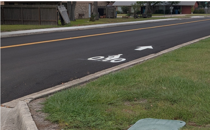
Bike lane on Smith Road in the process of being striped Source: City of Port Lavaca
