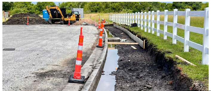
Construction on Smith Road to add sidewalks and bike lanes. Source: City of Port Lavaca
