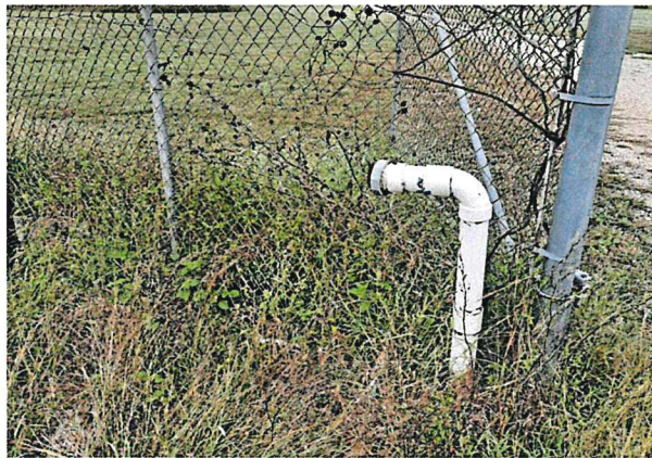
No. 7 Parcel 3 - Piping stick-up near back gate
