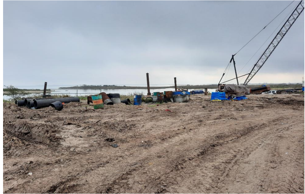
No. 2 Graded area and drum storage. Crane in use to place dock structure.
