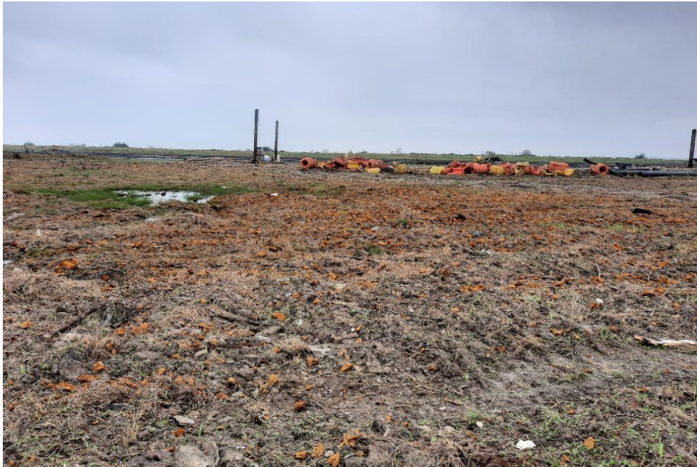
No. 9 Graded area - extensive orange foam debris
